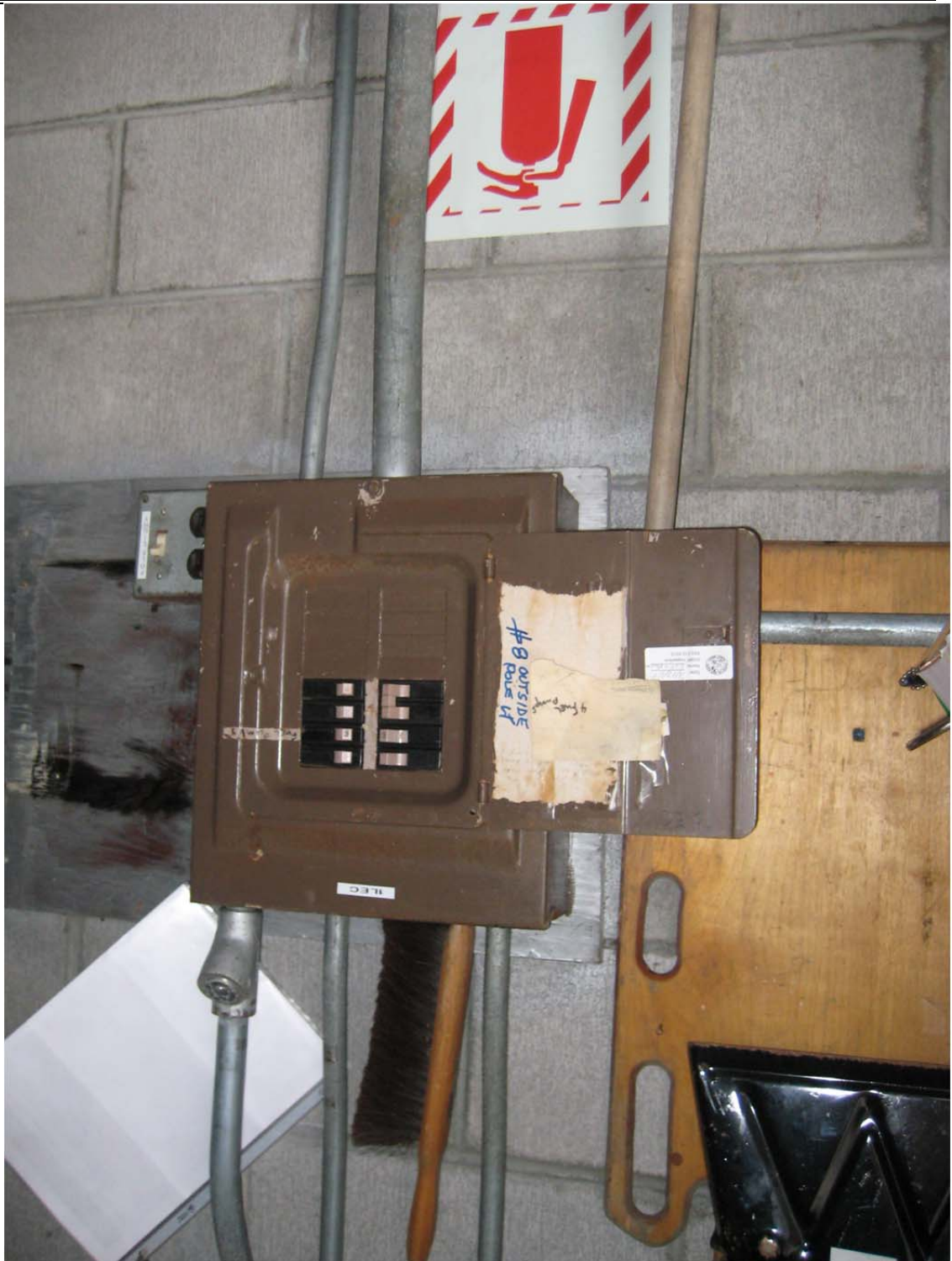
EE4 – Storage Room panel
