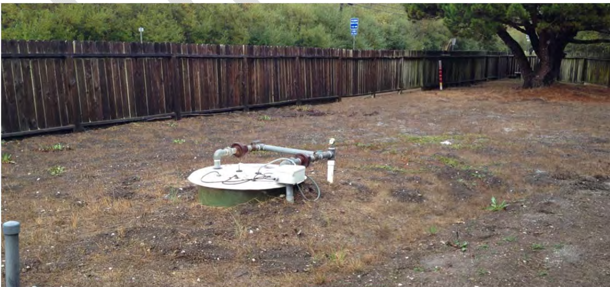
Septic field with flood elevation marker (white post with red marks) shown in the background
