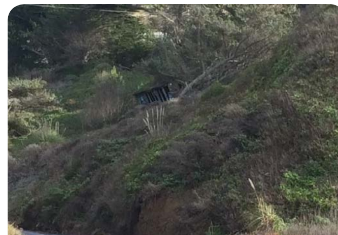
EROSION NEAR TUNITAS CREEK
