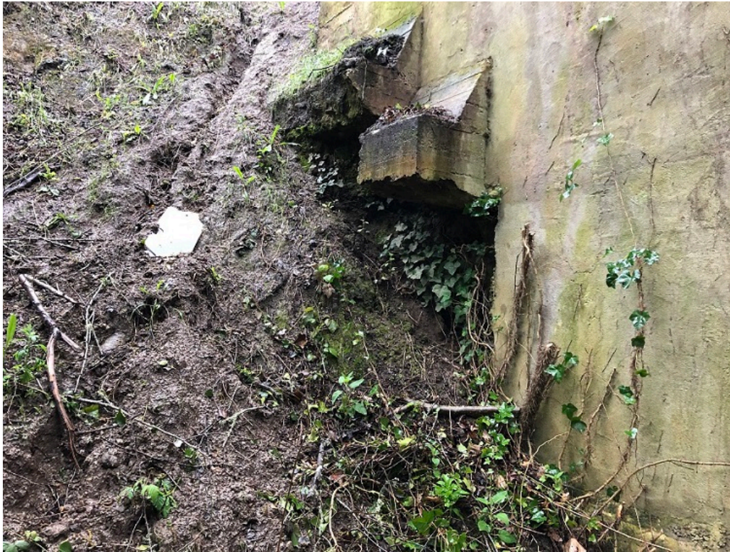
View of the undermined portion of the southeast wingwall.
