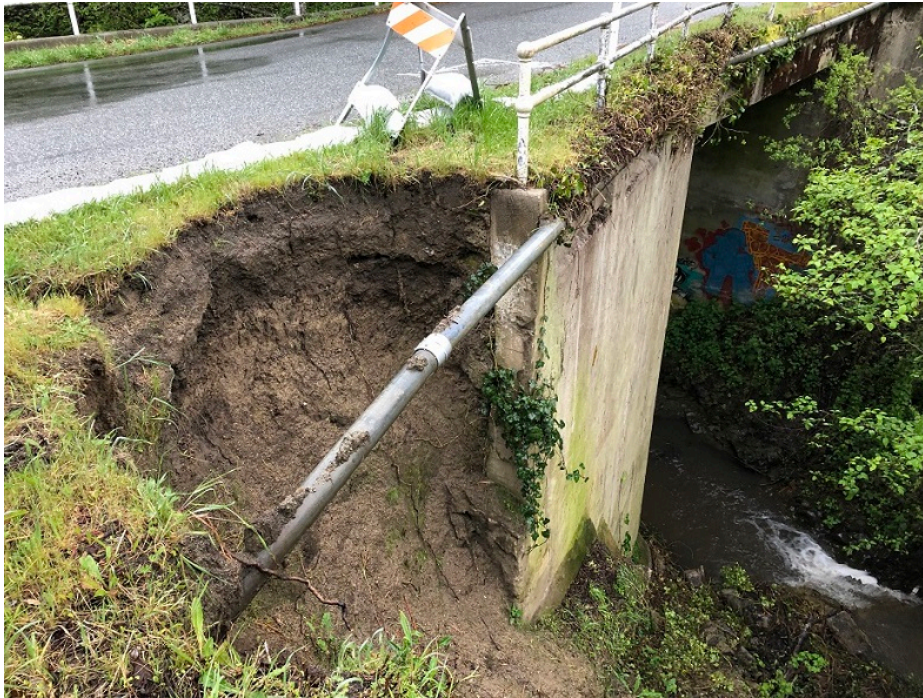
View of the landslide looking down from the south roadway shoulder. Note the exposed communication conduit.
