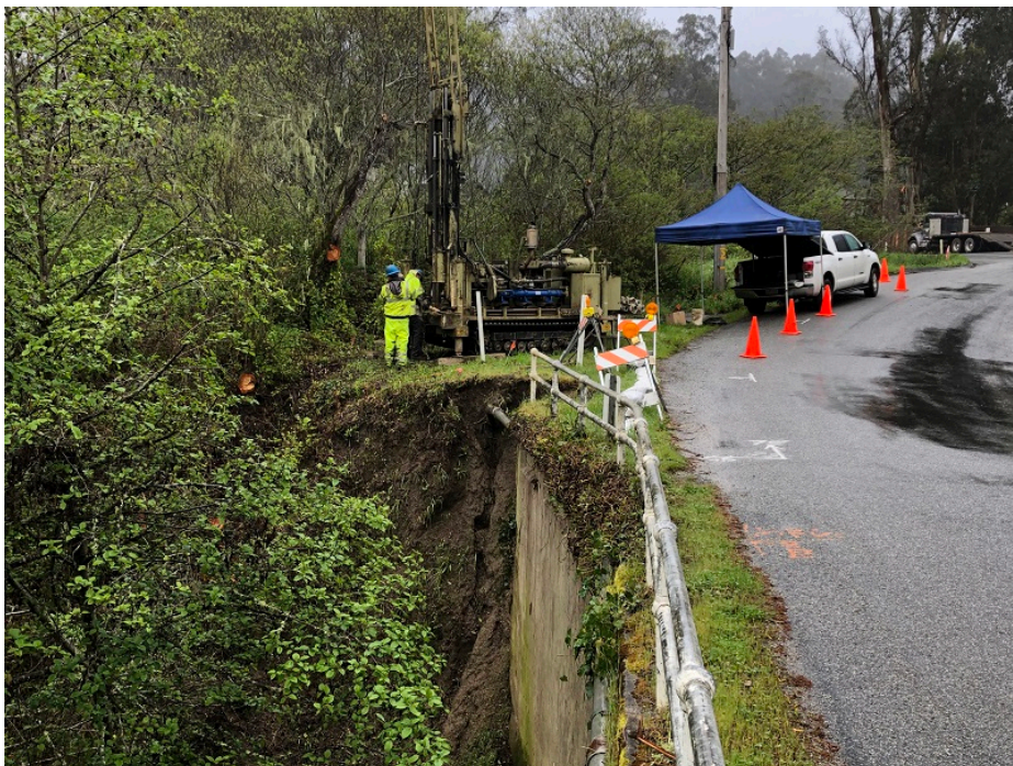
View of the landslide looking south along the roadway.
