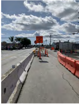
Temporary sidewalk / Acera temporal
