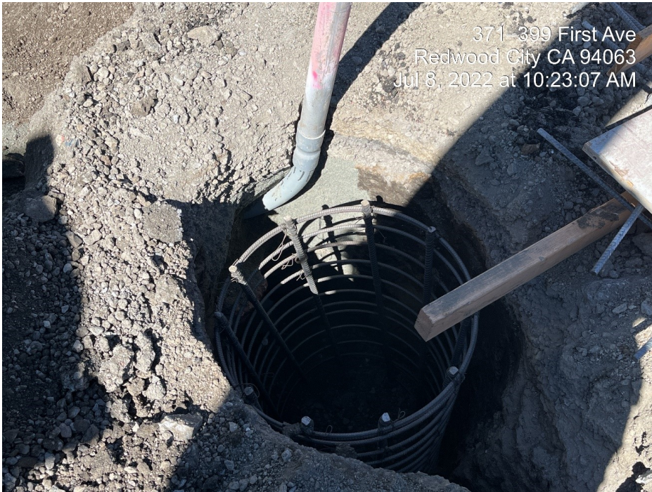
Street Light Foundation
