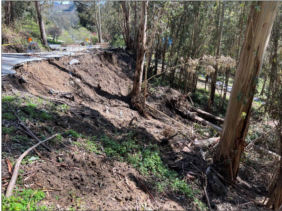
Photo 5: General southeast-facing view of slide area along the outboard edge of Higgins Canyon Road. Photo was taken during our last site visit on March 20 th , 2023.
