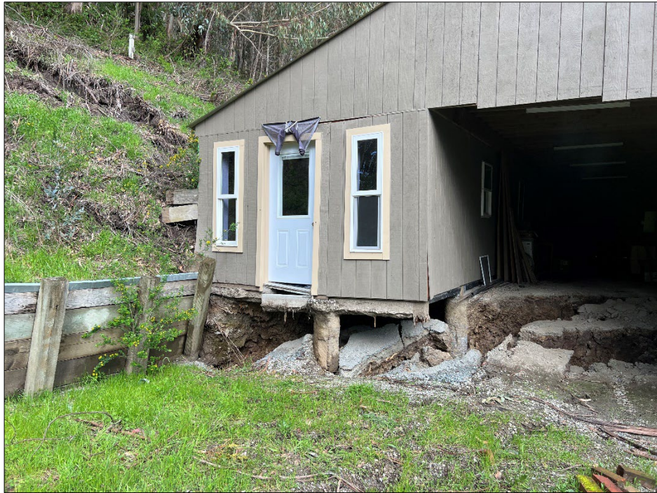
Photo 15: Northeast-facing view of the main scarp exposed beneath the barn on the upslope private property at (2175 Higgins Canyon Road). Note the main landslide scarp continues upslope after cutting beneath the barn. Also, note exposed barn foundation piers. Photo was taken during our last site visit on March 20 th , 2023.
