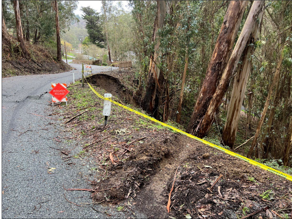
Photo 1: View of first slip-out (facing southeast) during our initial site visit on January 10 th , 2023.
