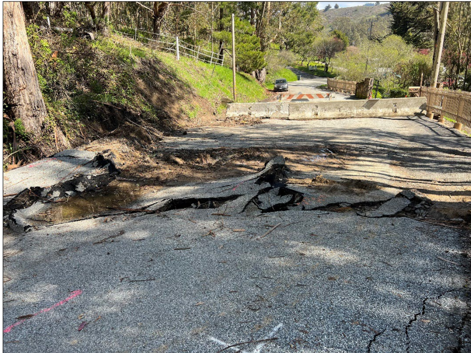
Photo 11: Buckling and thrusting of Higgins Canyon Road pavement near the inboard edge of the road and at the eastern extent of the road deformation. Photo was taken during our last site visit on March 20th, 2023.
