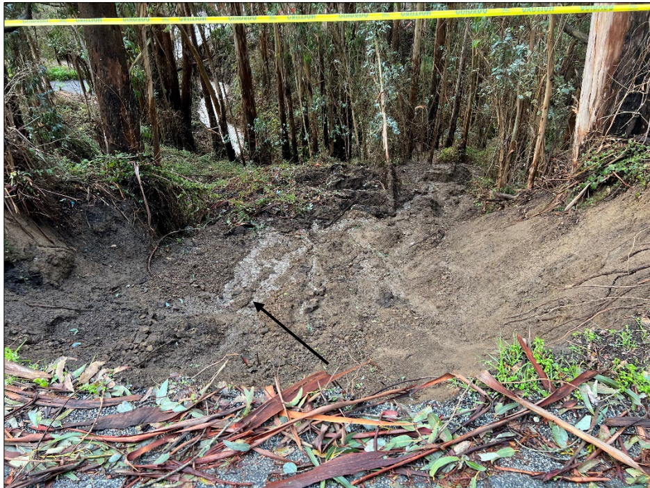
Photo 4: Southwest-facing view of the slip-out downslope of Higgins Canyon Road. Several seepage areas were observed along the base of the scarp (see black arrow). Photo was taken during our initial site visit on January 10th, 2023.
