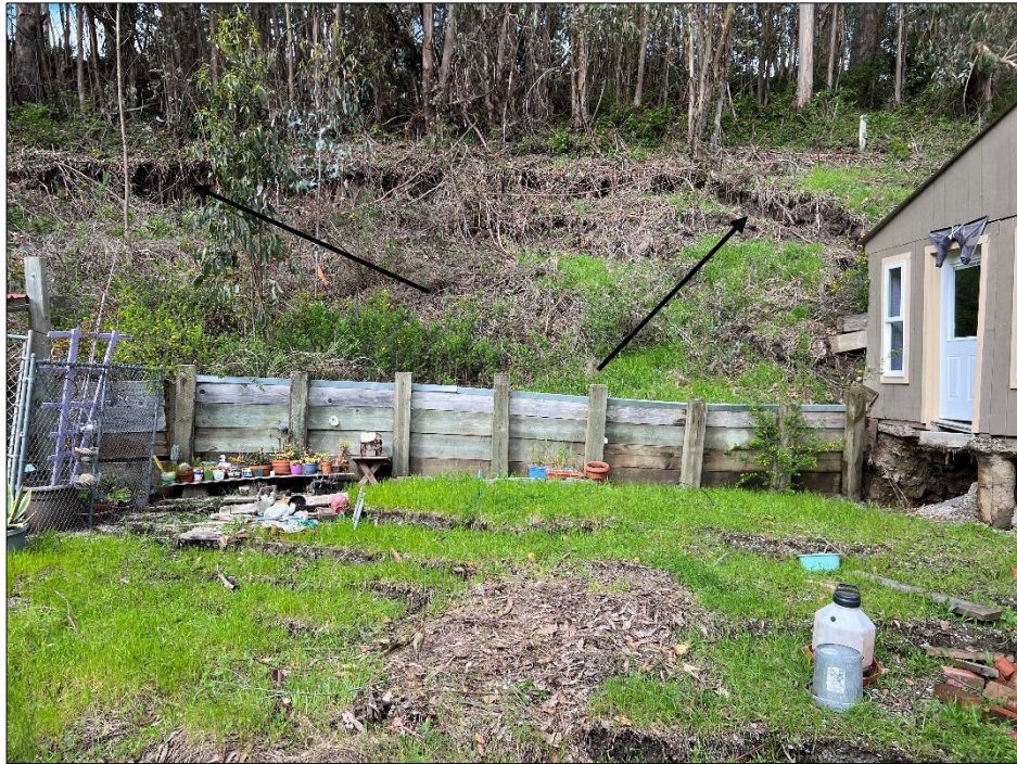
Photo 13: Northeast-facing view of the retaining wall on the upslope private property at (2175 Higgins Canyon Road). Note the main landslide scarp exposed upslope of the retaining wall. Also note tension cracks in the grass in front of the retaining wall. Photo was taken during our last site visit on March 20 th , 2023.
