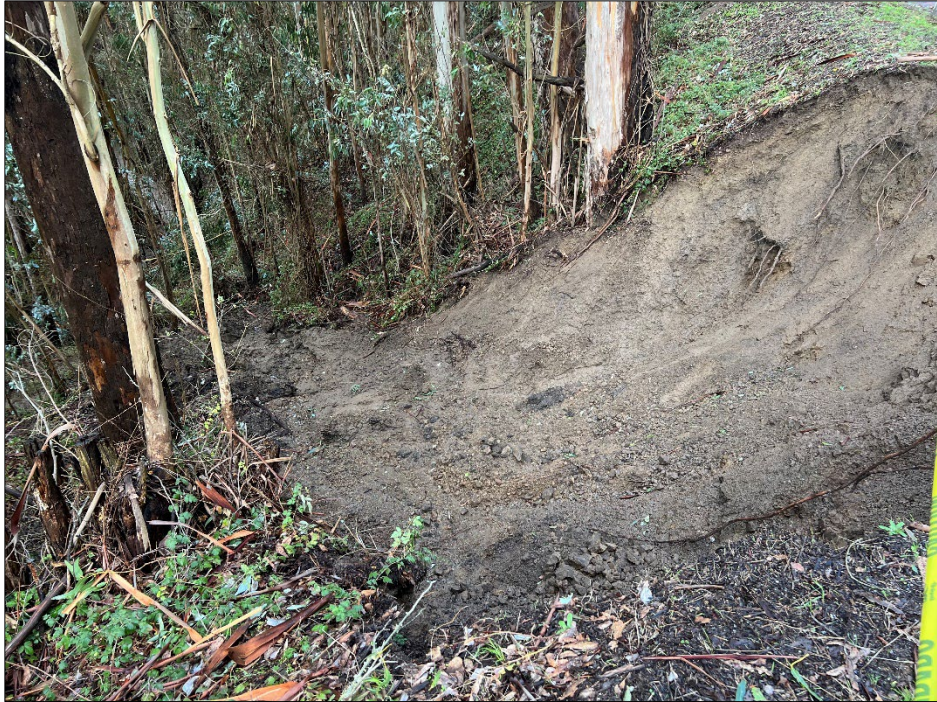
Photo 3: West-facing view of the downslope extent of the original slip-out along the outboard edge of Higgins Canyon Road. Photo was taken during our initial site visit on January 10th, 2023.
