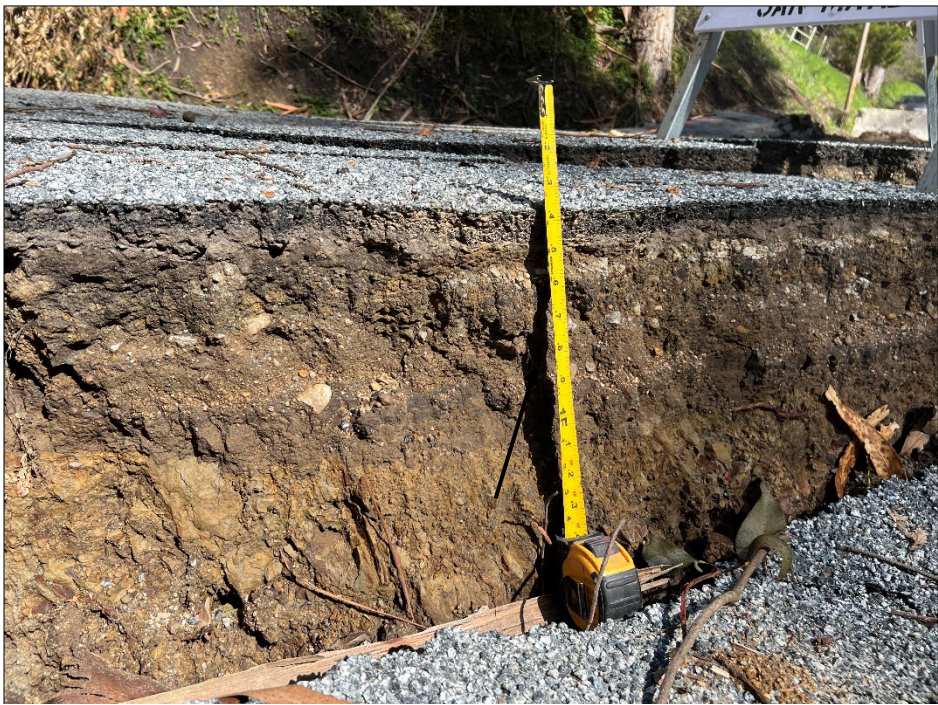
Photo 8: Approximately 13 inches of vertical displacement in Higgins Canyon Road pavement. Photo was taken during our last site visit on March 20th, 2023.
