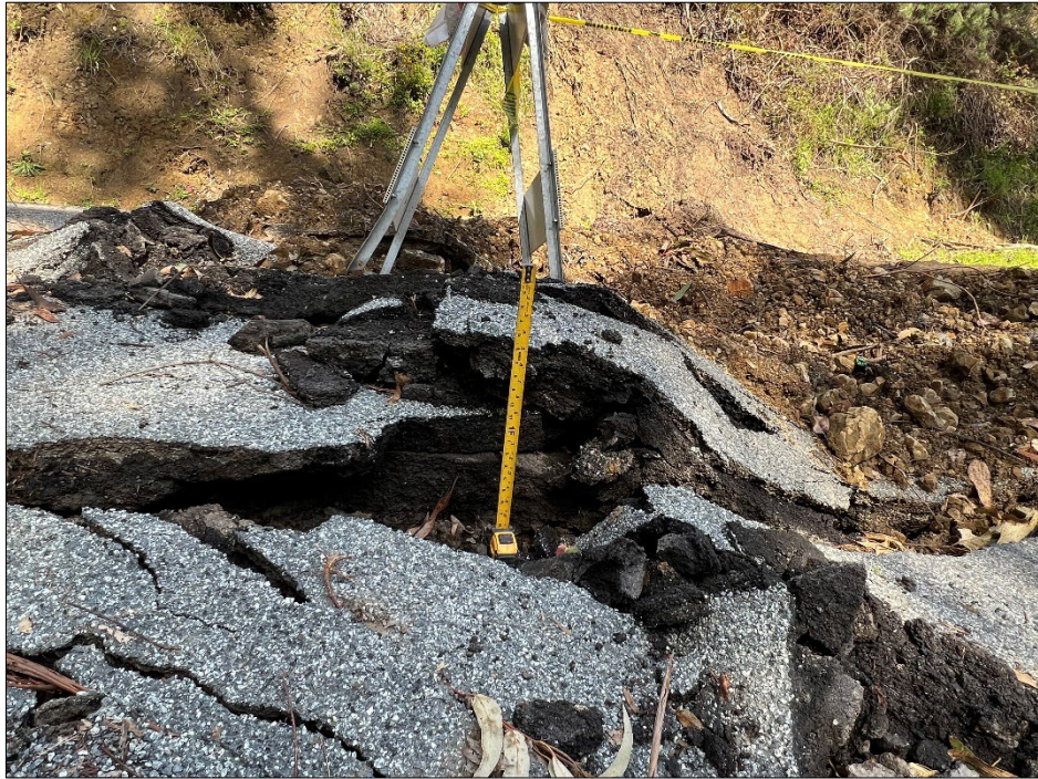
Photo 9: Vertical displacement in Higgins Canyon Road pavement due to buckling and thrusting. Photo was taken during our last site visit on March 20th, 2023.
