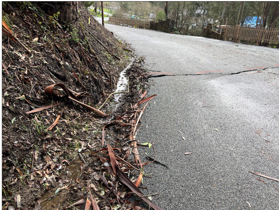
Photo 10: Southeastern extent of road deformation expressed as a crack with left lateral movement during our initial site visit on January 10 th , 2023.
