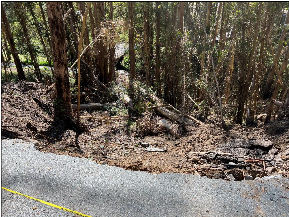
Photo 6: General southwest-facing view of slide area and fallen trees along the outboard edge of Higgins Canyon Road. Photo was taken during our last site visit on March 20 th , 2023.
