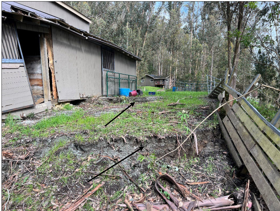
Photo 16: East-facing view of the northeastern extent of the slide deformation on the upslope private property at (2175 Higgins Canyon Road). Photo was taken during our last site visit on March 20 th , 2023.
