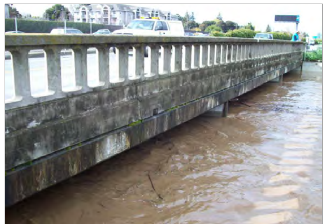
Flooding along San Francisquito Creek.
