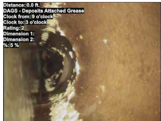
4, 00:01:11, 0.00ft Deposits Attached Grease, 35% of cross sectional area from 9 o'clock to 3 o'clock, within 8 inch, Start
