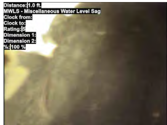
4, 00:00:47, 1.00ft Miscellaneous Water Level, Sag, 100% of the vertical dimension, Start
