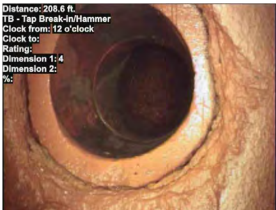
29, 00:12:37, 208.60ft Tap Break-in/Hammer at 12 o'clock, dia/height: 4.000inch
