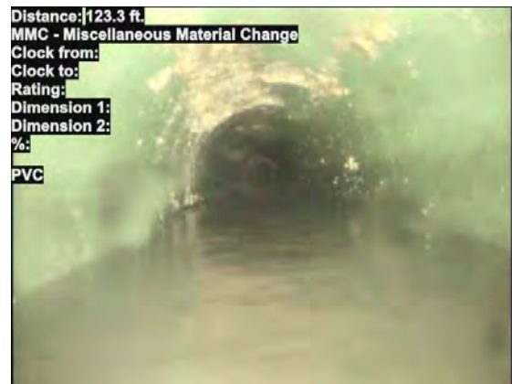
16, 00:13:47, 123.30ft Miscellaneous Material Change / PVC
