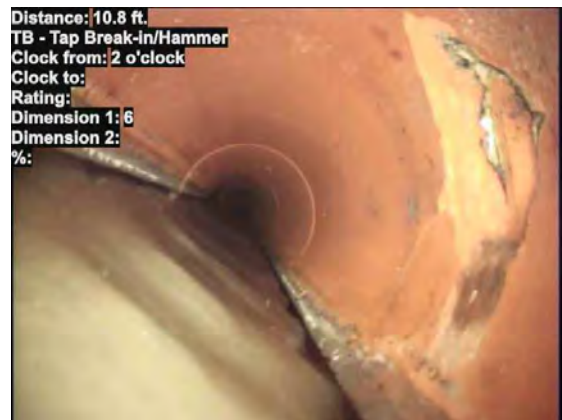
4, 00:01:17, 10.80ft Tap Break-in/Hammer at 2 o'clock, dia/height: 6.000inch, within 8 inch
