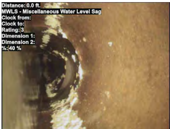
3, 00:00:43, 0.00ft Miscellaneous Water Level, Sag, 40% of the vertical dimension, Start
