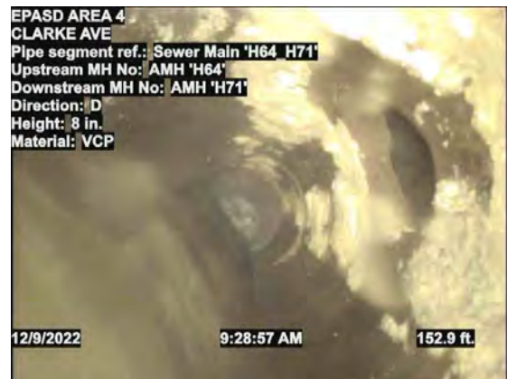
22, 00:15:31, 152.80ft Tap Break-in/Hammer at 2 o'clock, dia/height: 4.000inch, within 8 inch
