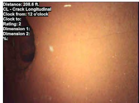
30, 00:13:11, 208.60ft Crack Longitudinal at 12 o'clock
