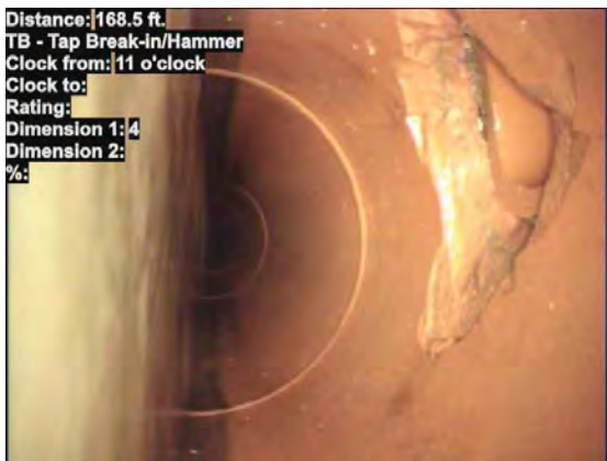
27, 00:10:43, 168.50ft Tap Break-in/Hammer at 11 o'clock, dia/height: 4.000inch
