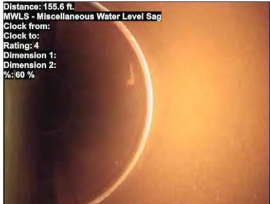
19, 00:08:49, 155.60ft Miscellaneous Water Level, Sag, 60% of the vertical dimension, Start
