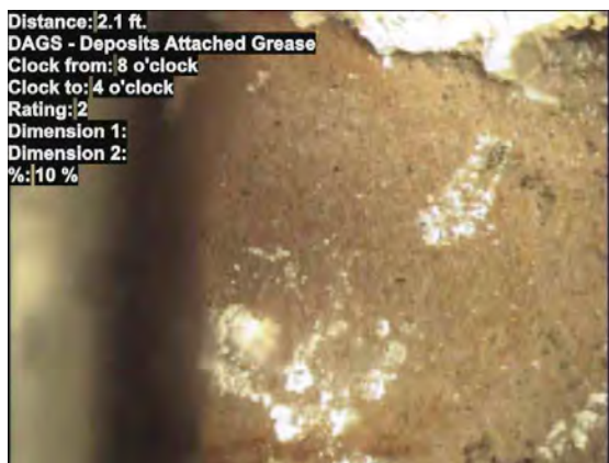
5, 00:01:09, 2.10ft Deposits Attached Grease, 10% of cross sectional area from 8 o'clock to 4 o'clock, Start
