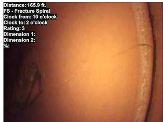
22, 00:09:42, 165.90ft Fracture Spiral from 10 o'clock to 2 o'clock, within 8 inch
