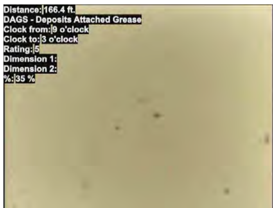
23, 00:18:15, 166.40ft Deposits Attached Grease, 35% of cross sectional area from 9 o'clock to 3 o'clock, within 8 inch, Finish
