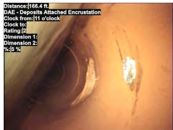
24, 00:10:13, 166.40ft Deposits Attached Encrustation, 5% of cross sectional area at 11 o'clock
