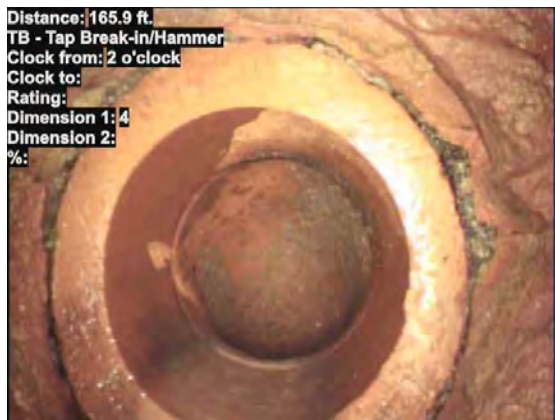
21, 00:09:27, 165.90ft Tap Break-in/Hammer at 2 o'clock, dia/height: 4.000inch, within 8 inch
