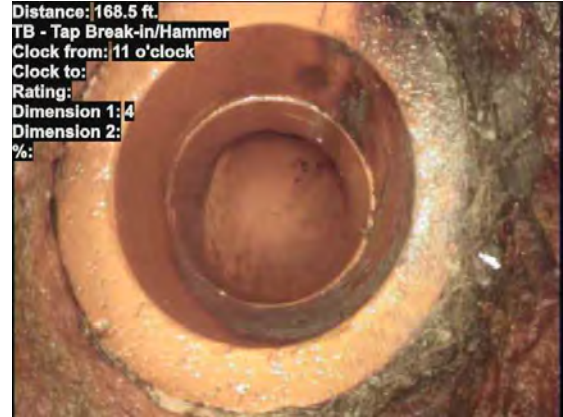
26, 00:10:43, 168.50ft Tap Break-in/Hammer at 11 o'clock, dia/height: 4.000inch
