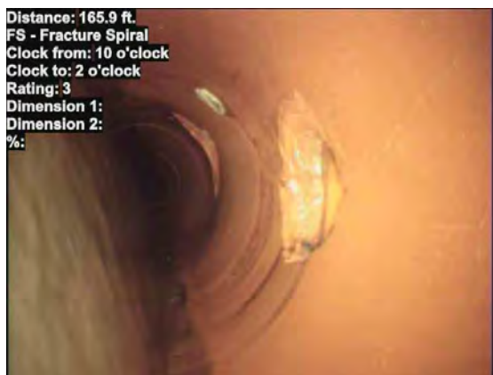
23, 00:09:42, 165.90ft Fracture Spiral from 10 o'clock to 2 o'clock, within 8 inch
