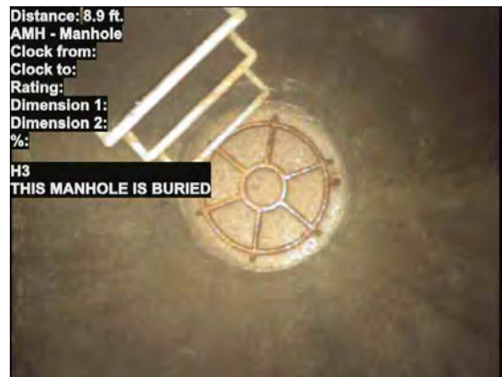
4, 00:01:34, 8.90ft Manhole / H3 THIS MANHOLE IS BURIED
