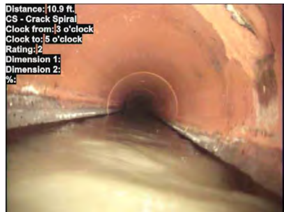
6, 00:01:46, 10.90ft Crack Spiral from 3 o'clock to 5 o'clock
