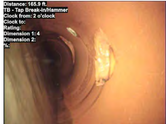
20, 00:09:27, 165.90ft Tap Break-in/Hammer at 2 o'clock, dia/height: 4.000inch, within 8 inch
