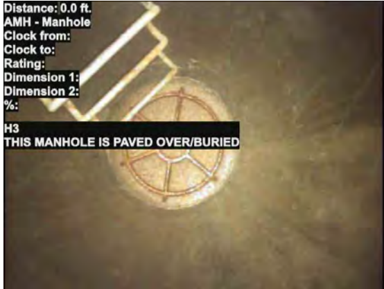
1, , 0.00ft Manhole / H3 THIS MANHOLE IS PAVED OVER/BURIED
