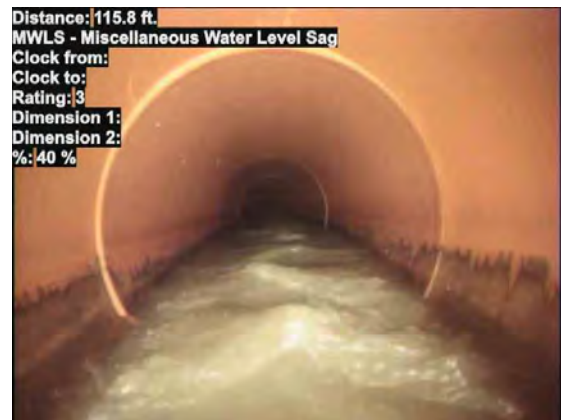
16, 00:07:12, 115.80ft Miscellaneous Water Level, Sag, 40% of the vertical dimension, Start
