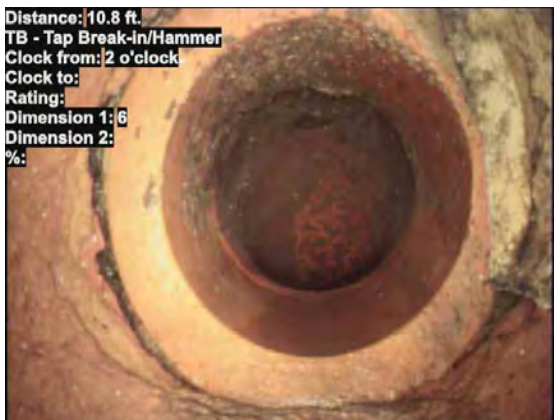
5, 00:01:17, 10.80ft Tap Break-in/Hammer at 2 o'clock, dia/height: 6.000inch, within 8 inch
