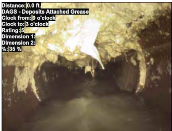
5, 00:01:11, 0.00ft Deposits Attached Grease, 35% of cross sectional area from 9 o'clock to 3 o'clock, within 8 inch, Start
