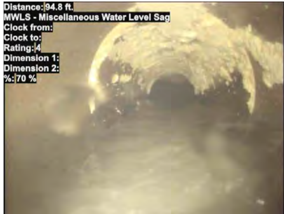
13, 00:12:24, 94.80ft Miscellaneous Water Level, Sag, 70% of the vertical dimension, Start
