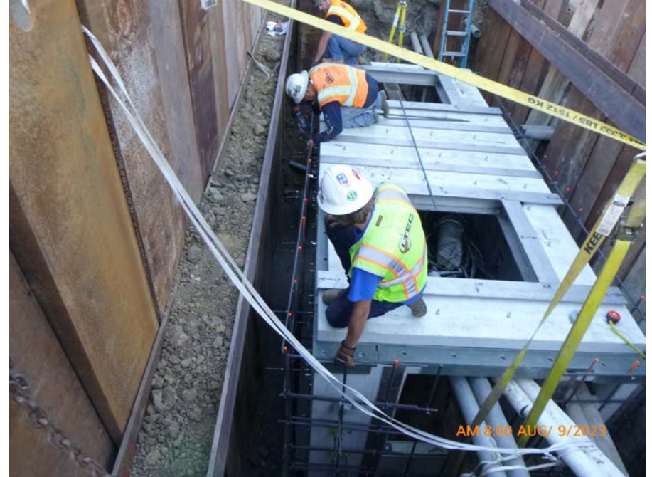
New AT&T Vault in Phase 5
