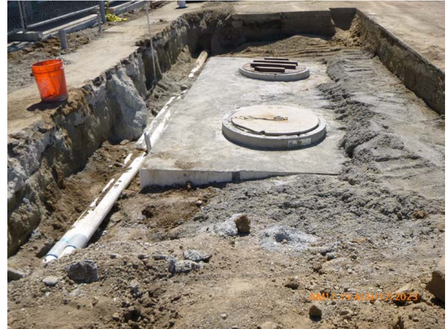
New AT&T Vault in Phase 5
