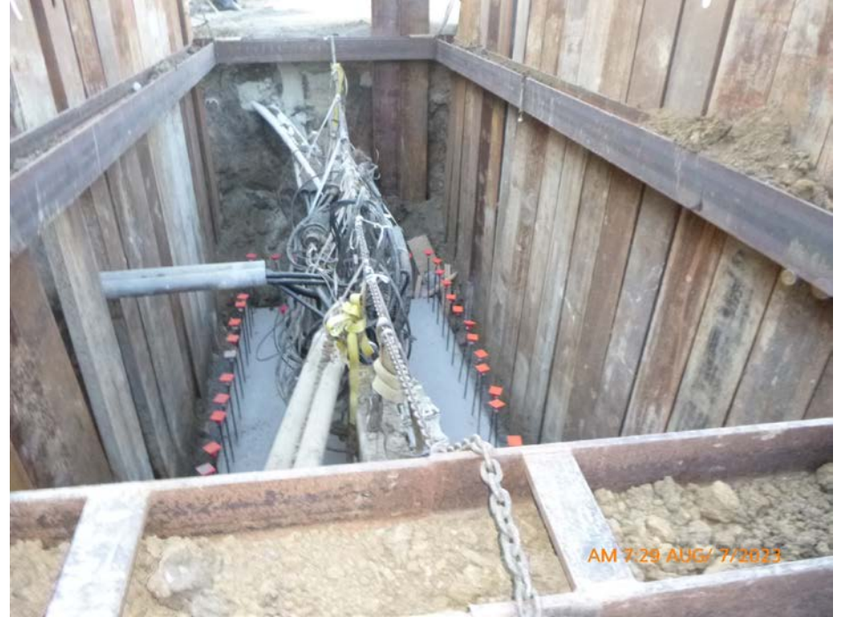
New AT&T Vault in Phase 5
