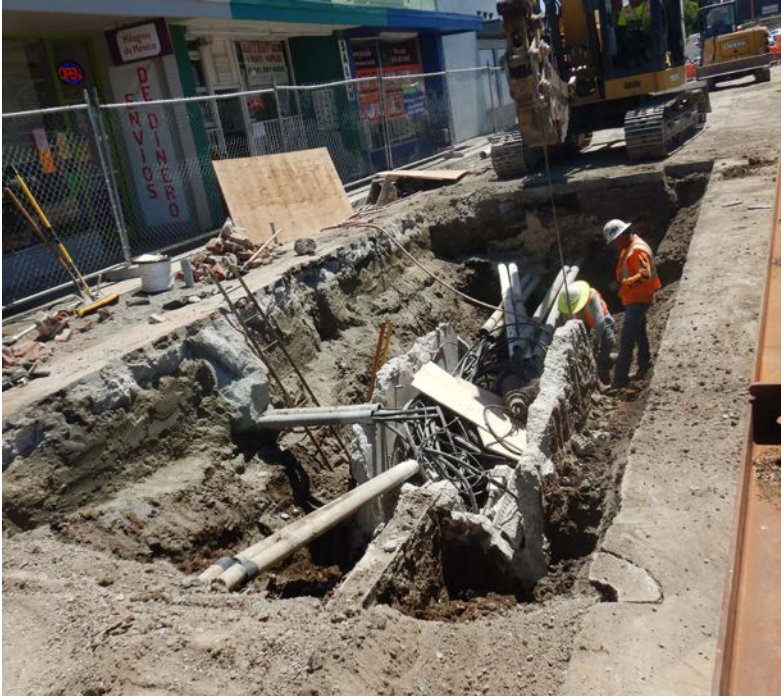
New AT&T Vault in Phase 5
