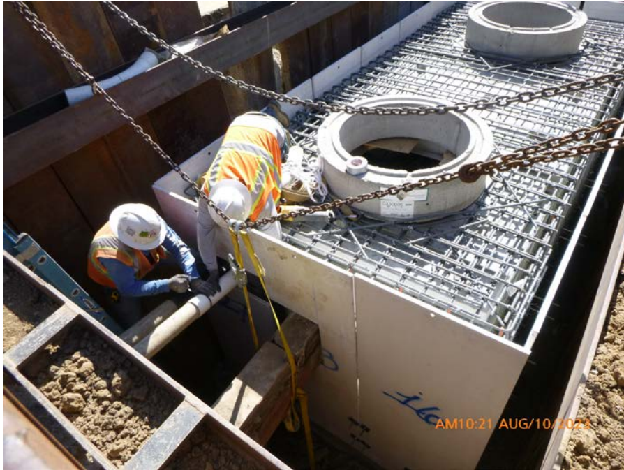
New AT&T Vault in Phase 5
