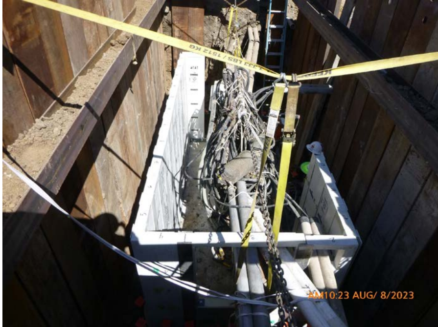
New AT&T Vault in Phase 5
