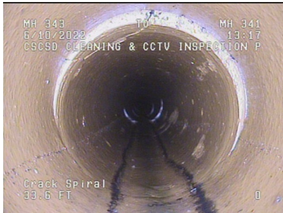
Example 1: Spiral Crack
