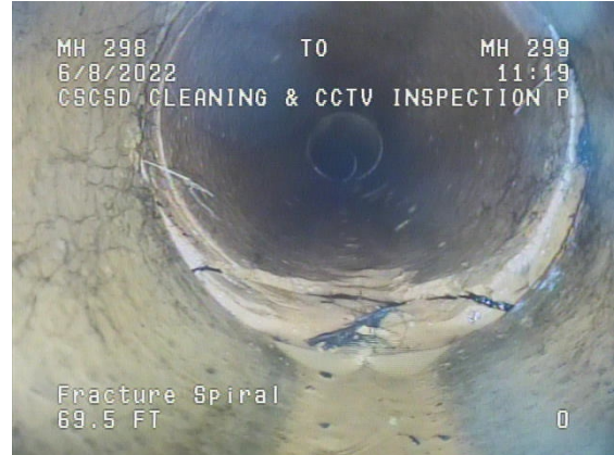
Example 4: Spiral Crack
