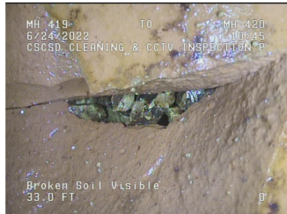
Example 10: Broken Pipe Soil Visible
