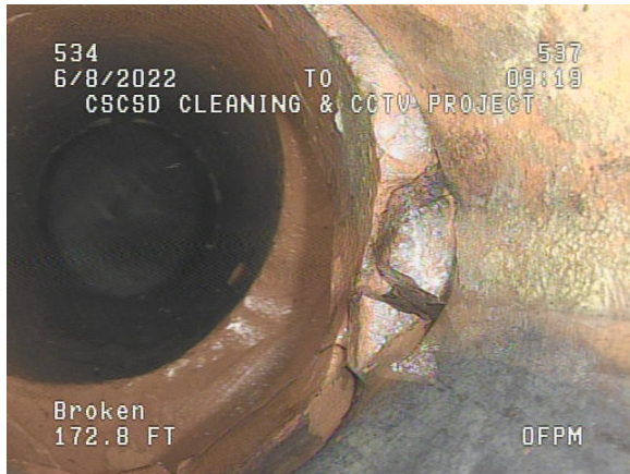
Example 7: Broken Pipe
