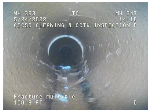
Example 6: Multiple Fractures
