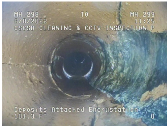
Example 3: Encrustation Deposits/Infiltration Stain
