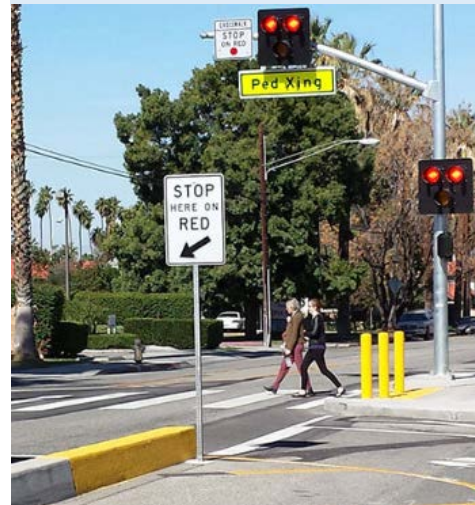
Pedestrian activated HAWK (High-Intensity Activated crosswalk)
