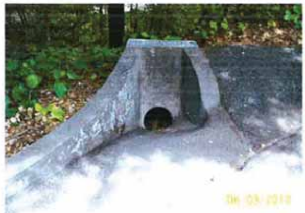
Figure 4. Adeline Drive. Drainage adjacent to 2888 Adeline Drive draining towards Mills Creek 500 feet below.
