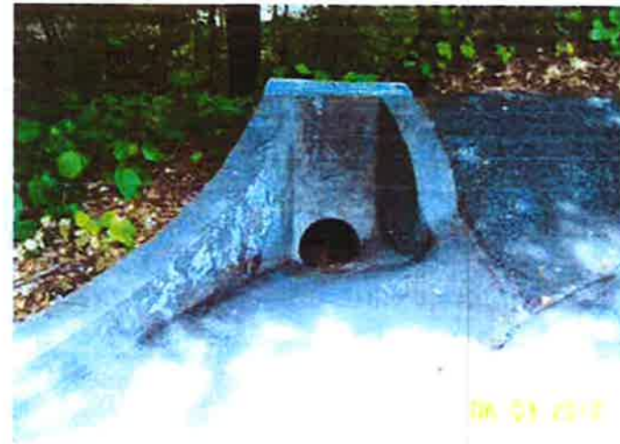
Photo 2. Adeline Drive. Drainage adjacent to 2888 Adeline Drive draining towards Mills Creek 500 feet below.
