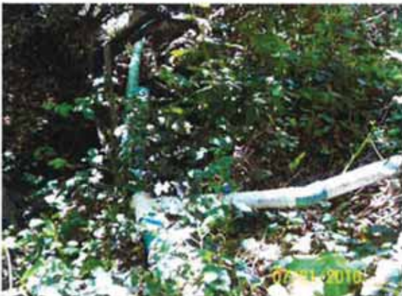
Figure 15. Newton Slide. Junction of temporary 4-inch spur line from 119 Los Robles drive to the temporary 6-inch main pipe.
