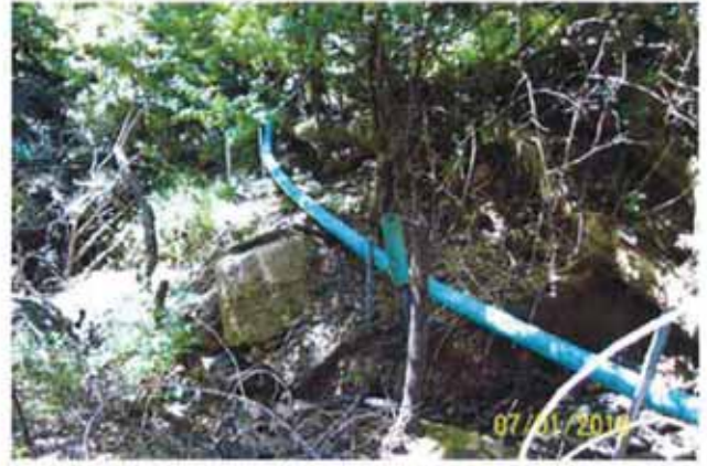
Figure 14. Newton Slide. Displaced manhole and sewer line due to slide activity required installation of temporary 6-inch pipe, running approximately 110 feet downslope to a downstream manhole.
