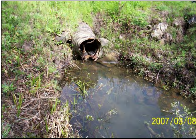
Photo 1. Deteriorated corrugated metal pipe (CMP) culvert located at Pigeon Point Road that requires replacement. (March 2007)
