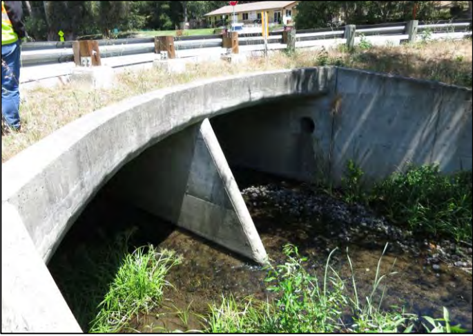
Photo 10. Concrete box culvert at Crystal Springs Road (near Polhemus Road) on San Mateo Creek. Potential maintenance needs include concrete patching of middle culvert wall. (May 2015)
