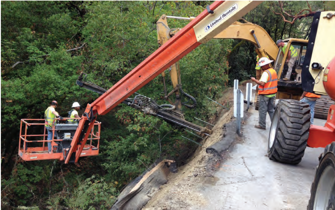
Photo 5. Example of soil nailing at a bank stabilization site along Alpine Road. (September 2014)
