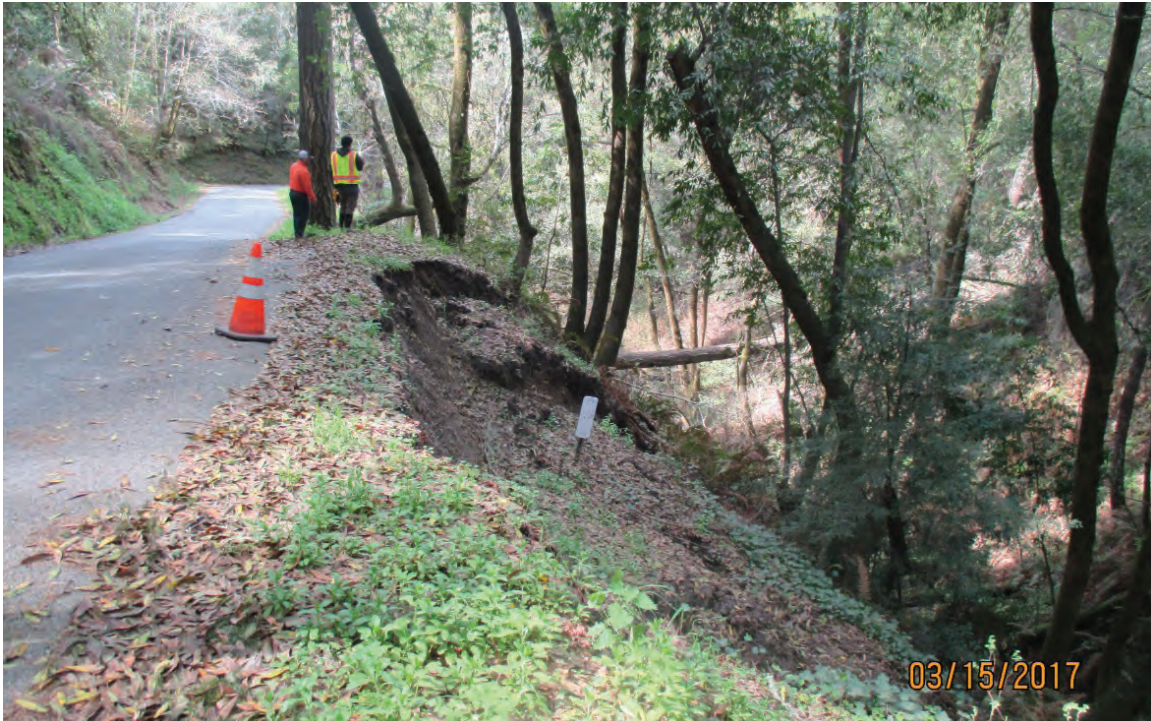
Photo 1. Example slope failure above unnamed tributary to Alpine Creek. This site was addressed in the County's 2017 emergency permit application. (March 2017)
