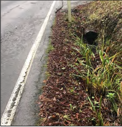
Photo 16. Example of an unpaved ditch and roadside culvert along Pescadero Creek Road and entrance to Sam McDonald Park. (December 2019)
