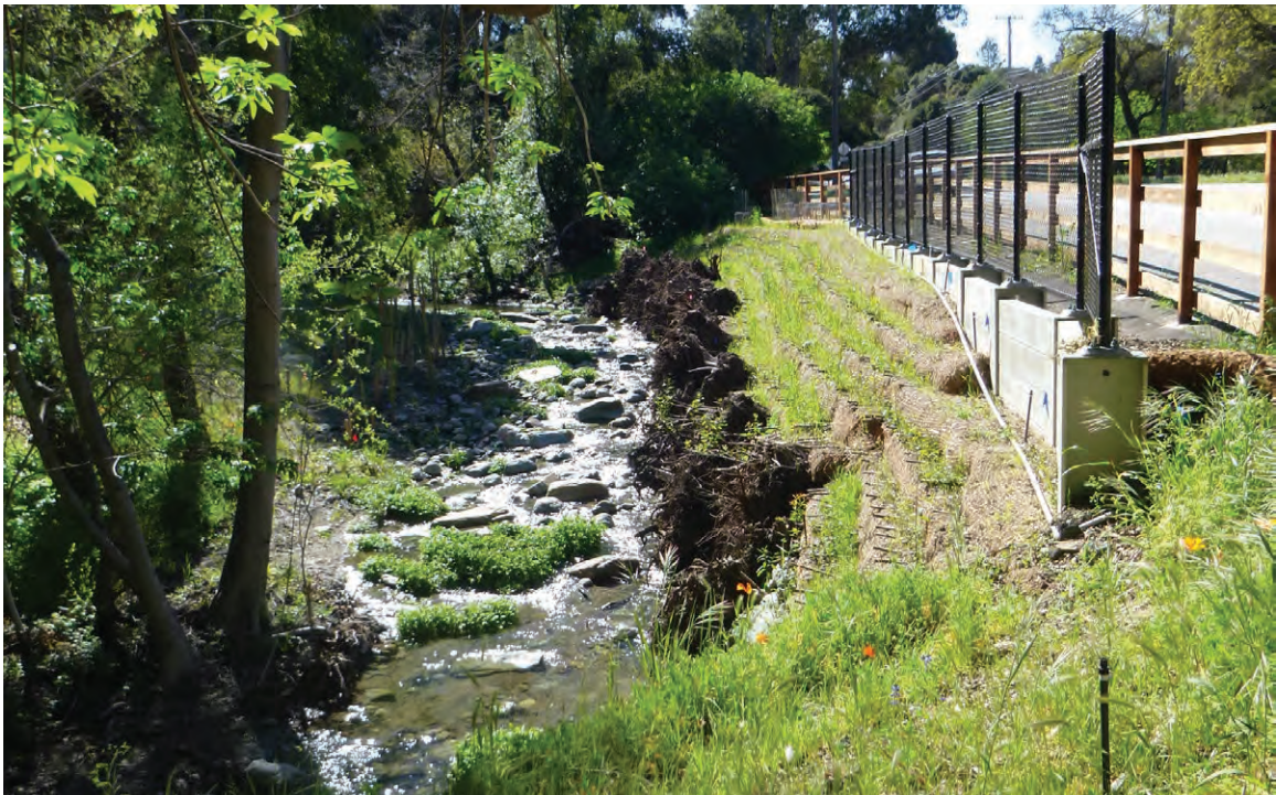
Photo 8. Example of a slider pile wall with grown-in vegetation at Los Trancos Rd. (March 2018)
