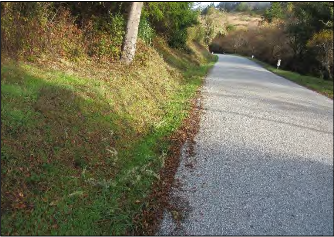
Photo 14. Another example of an inboard unpaved ditch along Gazos Creek Road. (December 2019)
