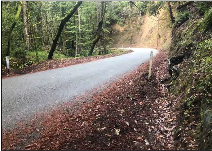
Photo 17. Example of an unpaved ditch along Alpine Road. (December 2019)
