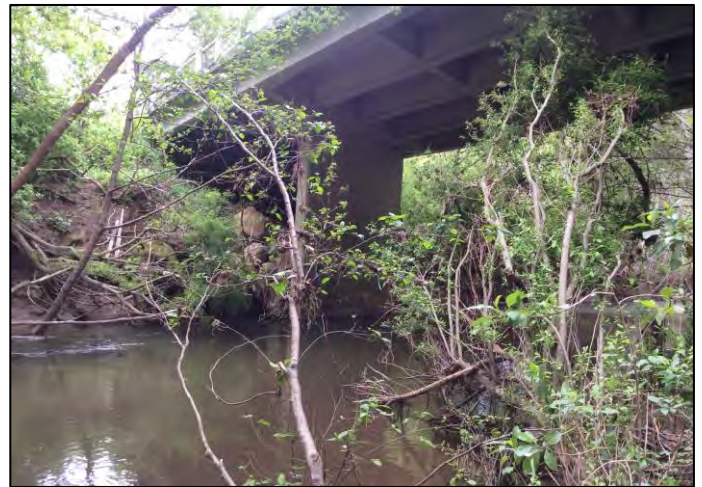
Photo 4. Pescadero Creek Road bridge near Cloverdale Road that requires routine maintenance including scour and erosion protection improvements at the base of the abutments. (April 2017)
