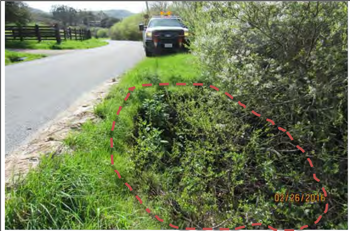
Photo 1 – Slip out location #1 (Red dashed line) on west side of Bear Gulch Road, looking north. (February 26, 2016)
