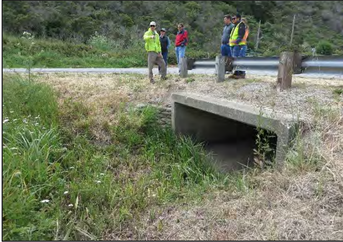
Photo 9. Concrete box culvert at Cloverdale Road and Butano Cutoff Road in Pescadero. Potential need for sediment and vegetation removal in the future. (May 2015)
