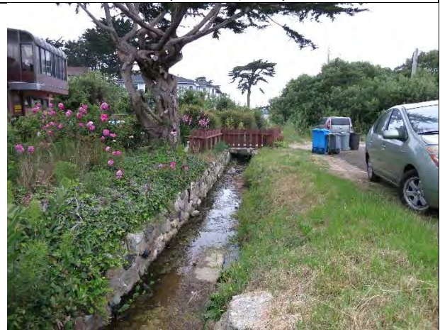
Photo 5. Looking downstream (west) along Kanoff Street. The ditch has a concrete bed while a rock revetment lines the left (south) bank. (March 18, 2015)
