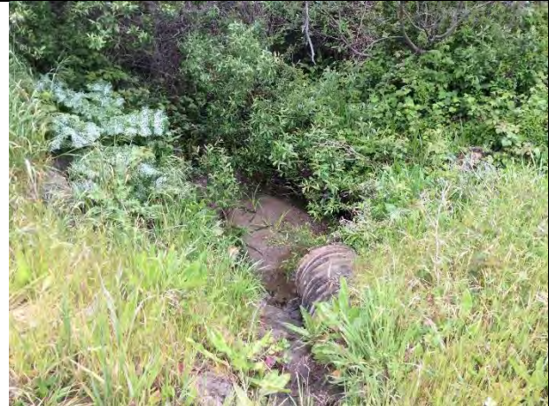
Photo 9. The downstream side of Mile 0.5 culvert. Sediment is deposited near the culvert outfall area before flows disperse over densely vegetated coastal scrub habitat. (April 6, 2017)
