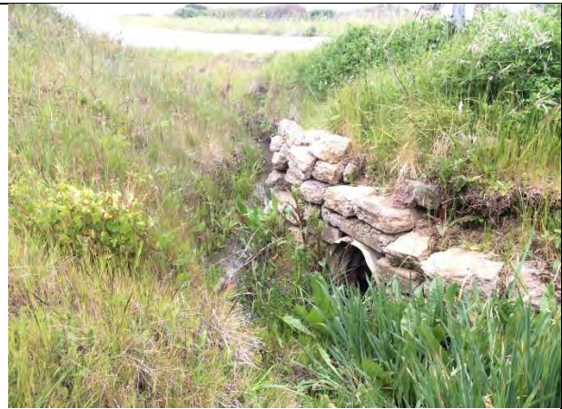
Photo 2. The upstream side of Mile 0.5 culvert. The culvert conveys surface runoff from Pigeon Point Road and a 600-foot (approximate) private driveway (April 6, 2017)
