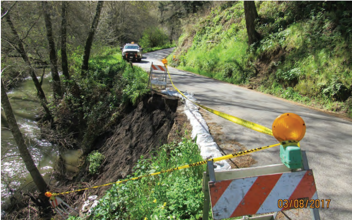
Photo 3. Example slope failure along Gazos Creek and Gazos Creek Road. This site was addressed in the County's 2017 emergency permit application. (March 2017)
