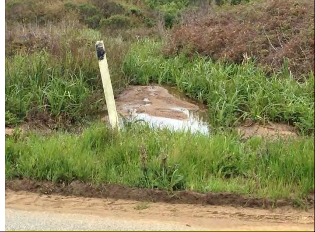
Photo 7. The downstream side of Mile 0.4 culvert. Sediment is deposited near the culvert outfall area before flows disperse over densely vegetated coastal scrub habitat. (April 6, 2017)
