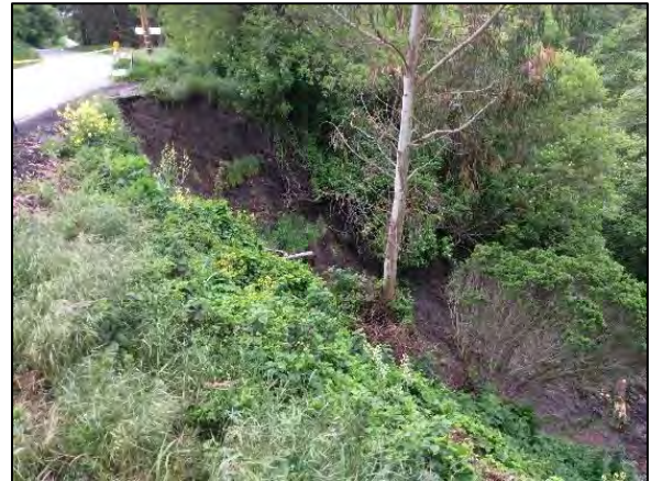
Photo 1. Bank slip-out along the north side of Tunitas Creek Road. (April 6, 2017)
