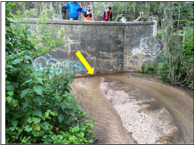
Photo 2. Upstream face of George Street bridge. The bridge culvert is nearly full of sediment (as indicated by the arrow). The reduced capacity has further decreased flow and resulted in a depositional area directly upstream of the bridge and formation of a large instream bar. (April 6, 2017)
