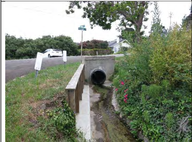
Photo 4. Culvert outfall on southwest corner of Kanoff Street. This portion of the drainage ditch along Kanoff Street is concrete. (March 18, 2015)
