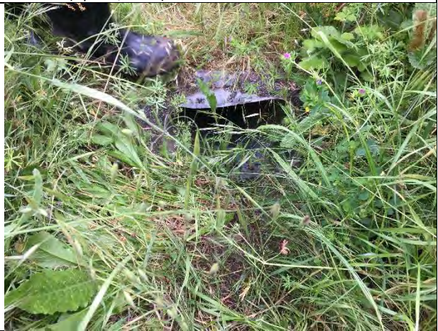
Photo 5. Failed culvert upslope from the bridge (April 6, 2017)
