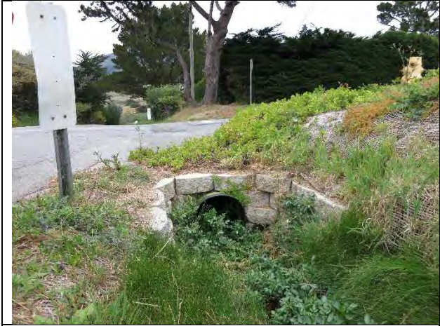
Photo 2. Culvert inlet on southeast corner of Farallone Avenue and 3 rd Street. (March 18, 2015)
