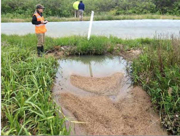
Photo 6. The upstream side of Mile 0.4 culvert. The culvert conveys stormwater runoff from the hillslope above. Sediment has accumulated at the culvert opening diminishing conveyance capacity. (April 6, 2017)
