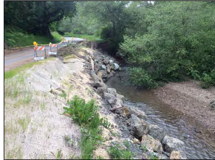
Photo 2. Gazos Creek in Pescadero. Photo shows a recent slip-out that occurred along Gazos Creek Road. (April 2017)
