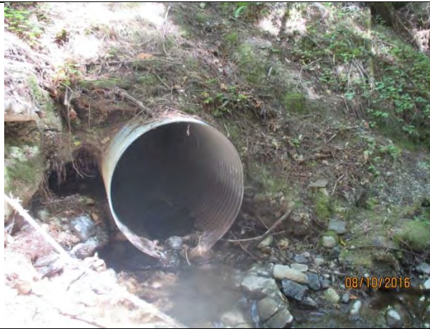
Photo 3. 0.9 Alpine culvert outlet (August 10, 2016).
