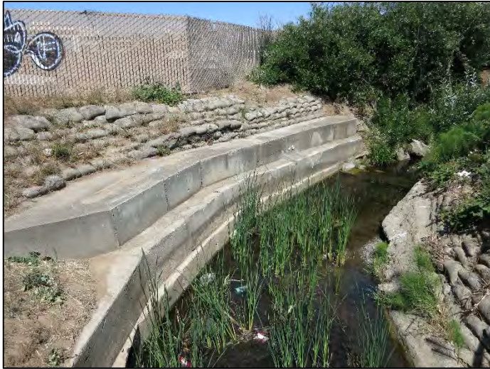
Photo 5. Belmont Creek downstream from Old County Road in Belmont, an example of a modified earthen channel (May 2015)
