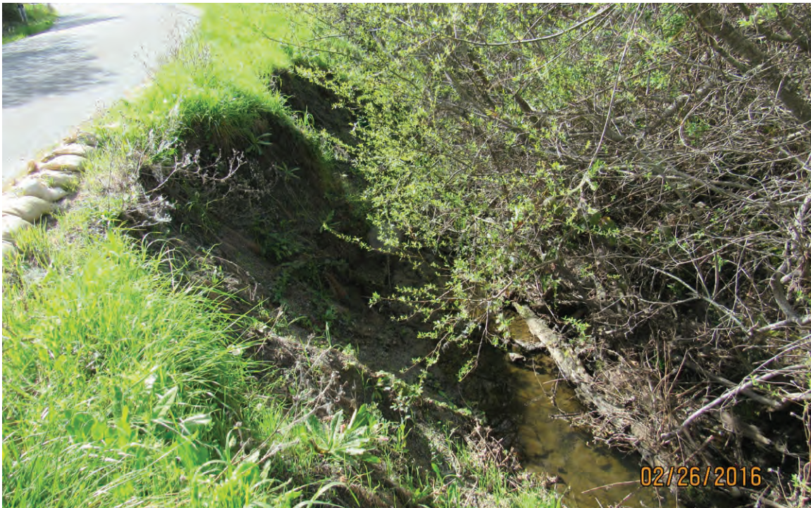
Photo 2. Bank failure along Lower Bear Gulch Road and adjacent to Clear Creek, an intermittent tributary to San Gregorio Creek. (February 2016)
