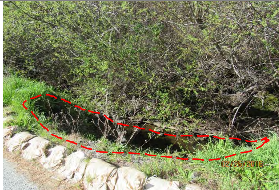
Photo 4- Slip out location #3. Edge of roadway and flowing water in Clear Creek pictured from Bear Gulch Road. (February 26, 2016)
