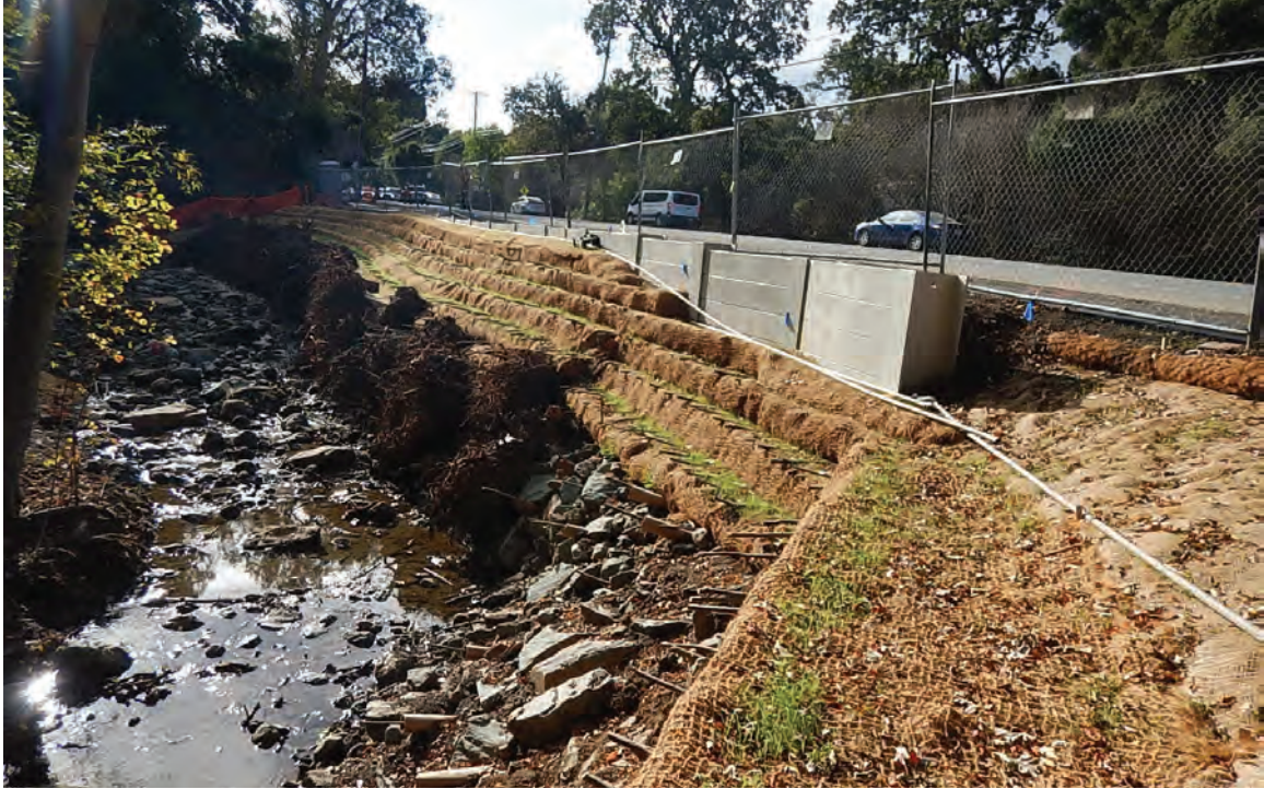
Photo 7. Example of a slider pile wall fronted with rock, rootwads, and vegetation following installation at Los Trancos Rd. (November 2017)
