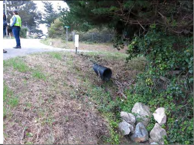
Photo 3. Culverted outfall at northwest corner of Farallone Avenue and 2 nd Street. (March 18, 2015)
