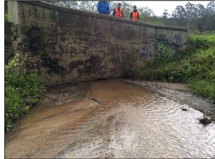
Photo 6. Upstream side of George Street bridge where substantial sediment accumulation has occurred and is blocking the culvert (April 2017)
