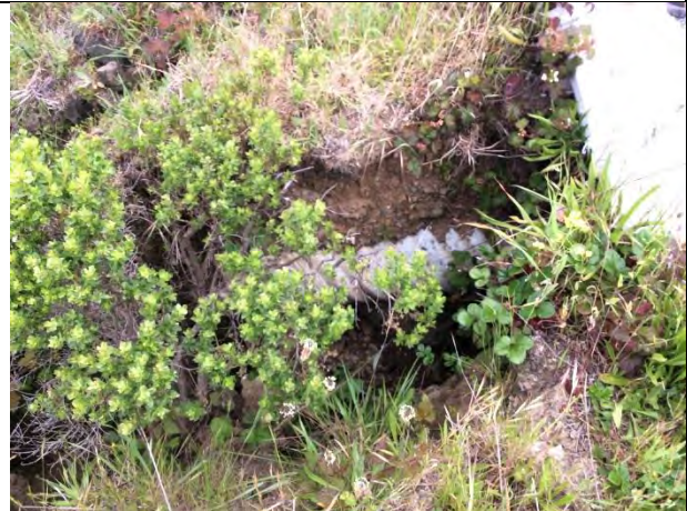
Photo 4. The upstream side of Mile 0.5 culvert. The culvert conveys surface runoff from Pigeon Point Road and a 600-foot (approximate) private driveway (April 6, 2017)
