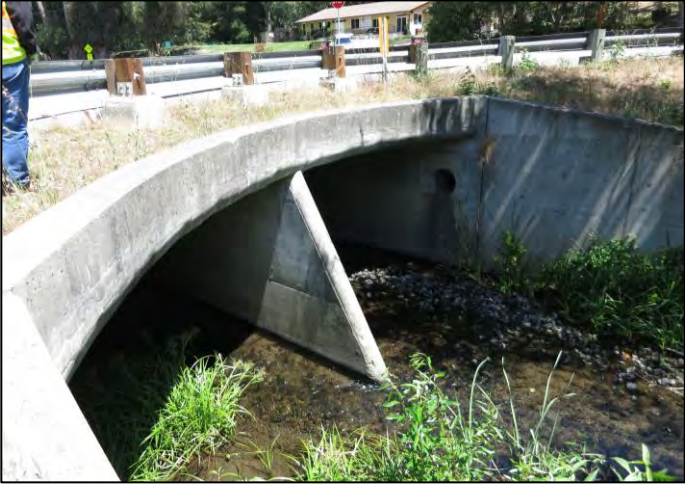
Photo 10. Concrete box culvert at Crystal Springs Road (near Polhemus Road) on San Mateo Creek. Potential maintenance needs include concrete patching of middle culvert wall. (May 2015)
