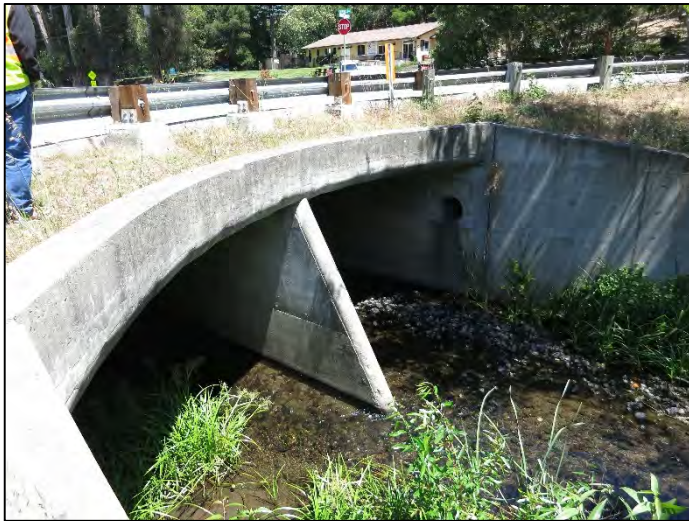
Photo 7. A concrete box culvert section of San Mateo Creek near Crystal Springs Road near its intersection with Polhemus Road (May 2017)
