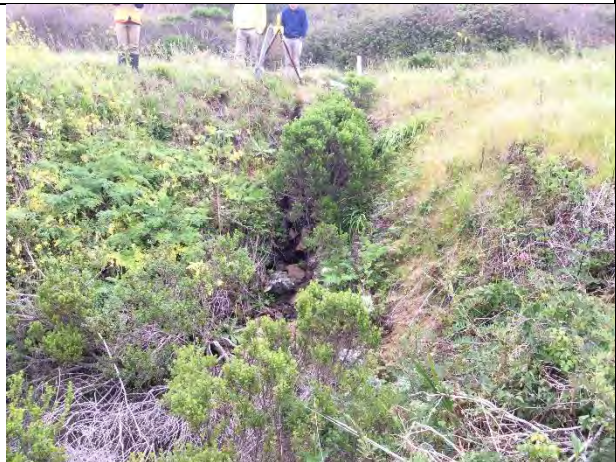
Photo 3. The downstream side of Mile 0.5 culvert. Sediment is deposited near the culvert outfall area before flows disperse under densely vegetated coastal scrub habitat. (April 6, 2017)
