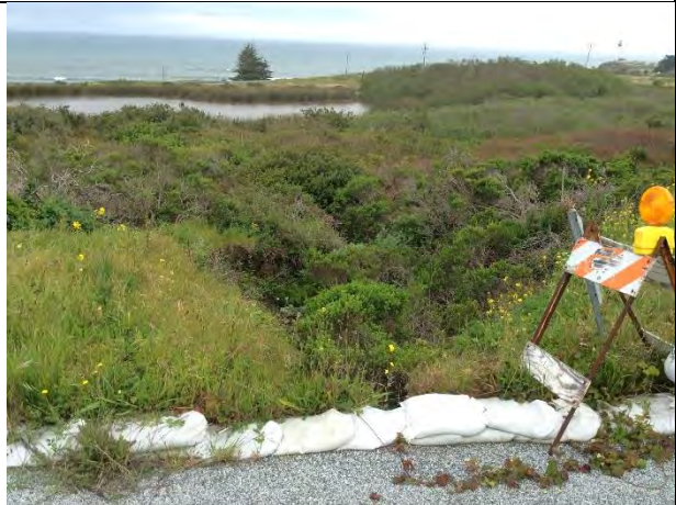
Photo 5. The downstream side of Mile 0.5 culvert. Sediment is deposited near the culvert outfall area before flows disperse under densely vegetated coastal scrub habitat. (April 6, 2017)
