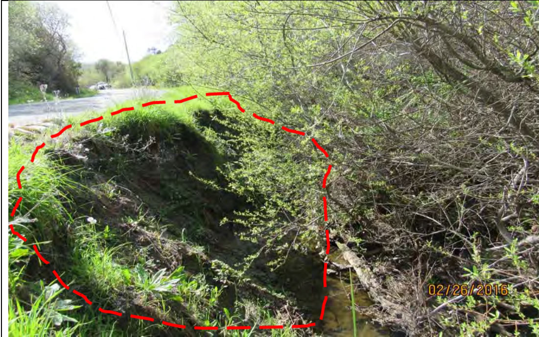
Photo 3. Slip-out Location #3 (Red dashed line) on the west side of Bear Gulch Road, looking south. (February 26, 2016)
