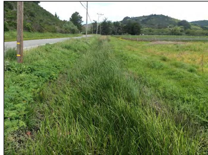
Photo 4. Earthen ditch adjacent to Cloverdale Road in Pescadero. (April 2017)
