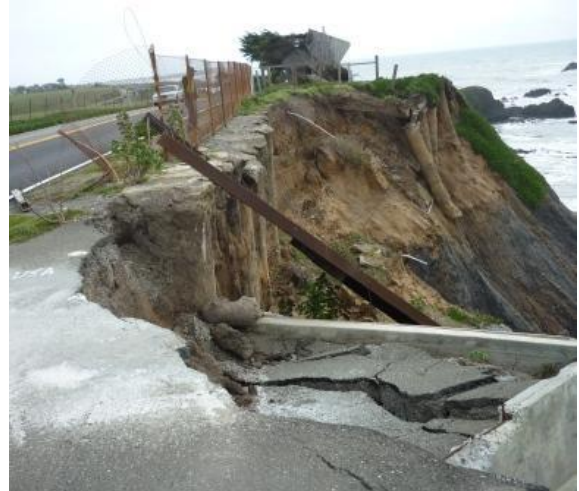
Coastal erosion along Highway 1 in Marin County
