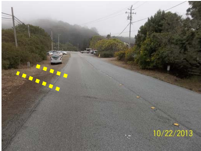
Photo 22 – Photo of Stage #1 project site. Dashed lines denote area of impact from construction activities. Excavation of culvert will begin at edge of pavement. Culvert drains neighboring property and roadside ditch into Palmer Gulch. A small sinkhole has developed at the point of culvert disconnection.
