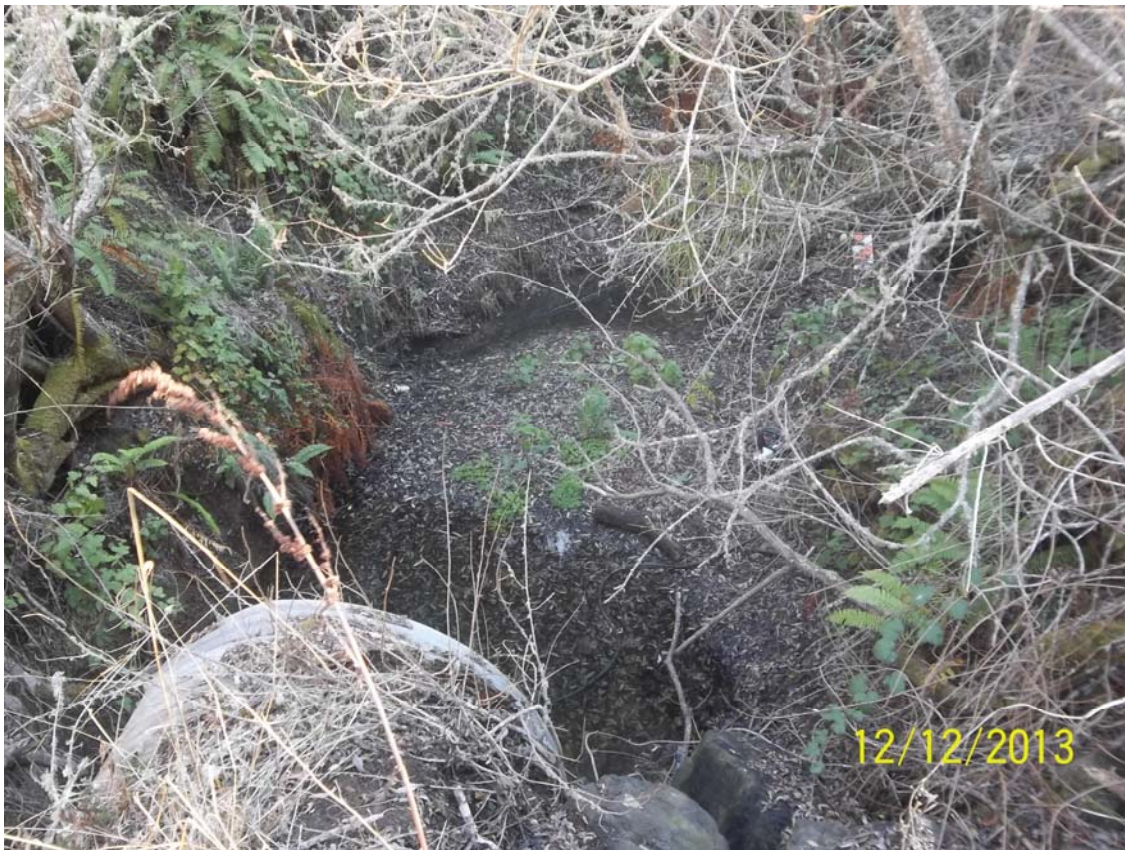
Photo 20 – Photo of culvert outlet pool and channel. The pool is expected to have negligible depth during the culvert replacement which will occur during the dry season. Substrate within the pool is mostly sand and silt with a heavy accumulation of leaf debris. No fish or wildlife were seen utilizing the pool during the site visits. Maximum pool depth at the time of the 12/12/2013 visit was approximately 1 foot.
