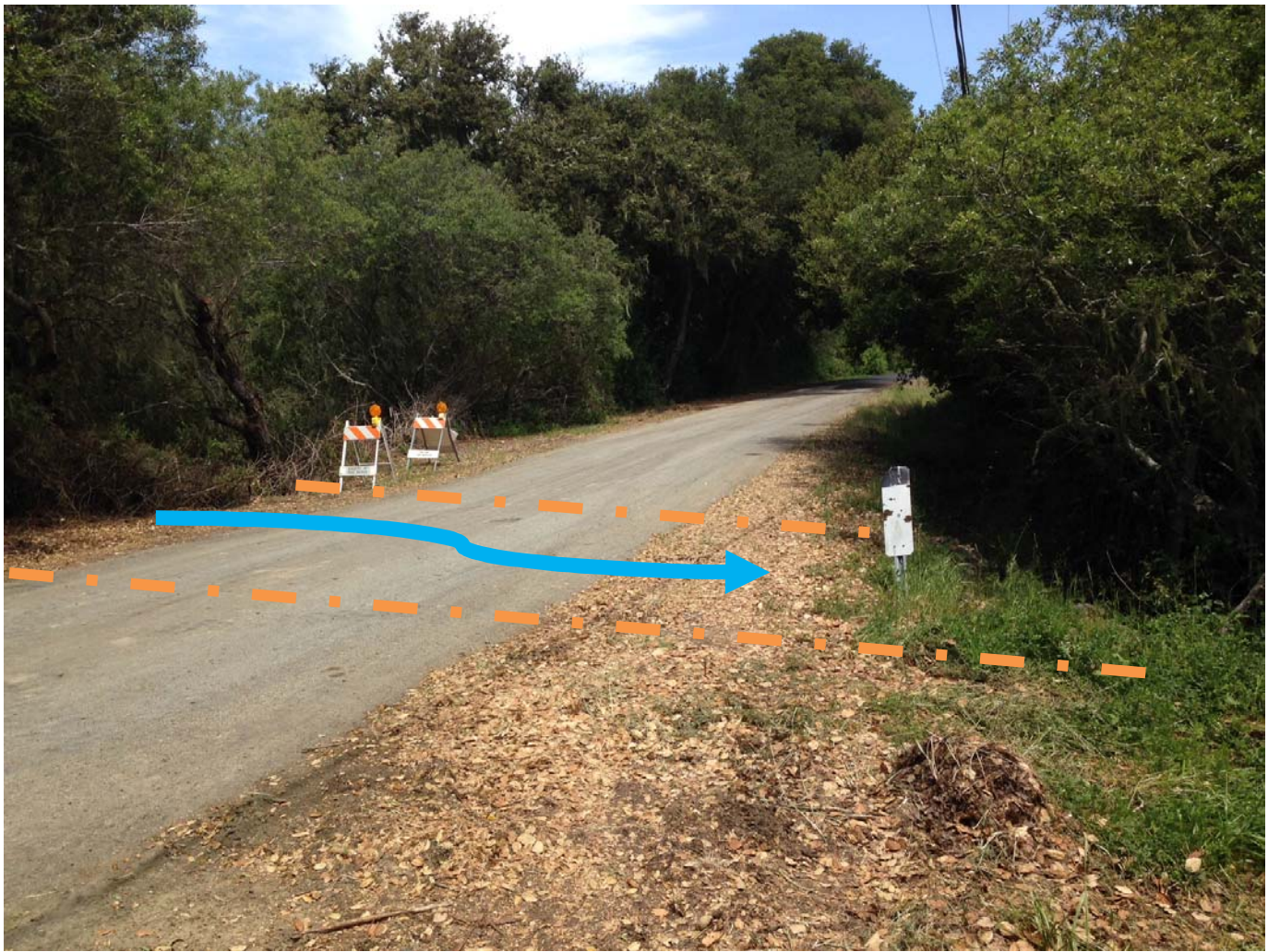
Photo 18 – Photo of Bear Gulch Road project site. Dashed lines indicate anticipated limits of project site activities. Traffic barricades identify sinkhole location. Roadside ditch exists on the east side of the road and drains into the culvert outlet plunge pool. Arrow indicates direction of stream flow. Construction will only take place when the site is dry and occur on one half of the road at a given time, leaving the other half of the road available for public egress and ingress.
