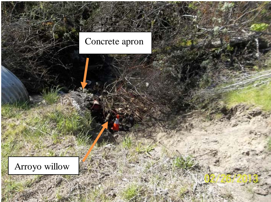
Photo 4 - Photo of the 36-inch CMP culvert outfall and the unnamed drainage. Slip-
