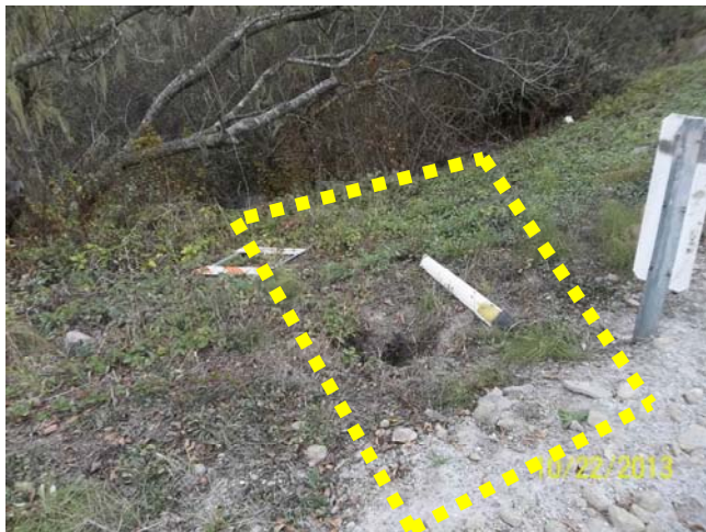
Photo 25 – Photo of culvert disconnection point and sinkhole. Sinkhole exists approximately 2 feet from the edge of pavement. Culvert outfall has a HDPE flume which directs water into the low gradient valley.
