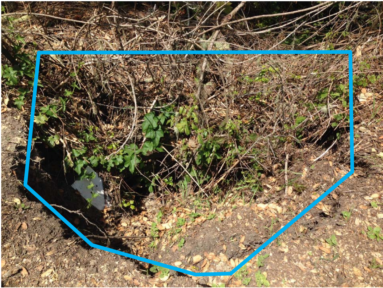
Photo 19 – Photo of sinkhole at culvert inlet caused by culvert disconnection. The hole is approximately 4 feet deep and 6 feet wide and is identified by the blue line.
