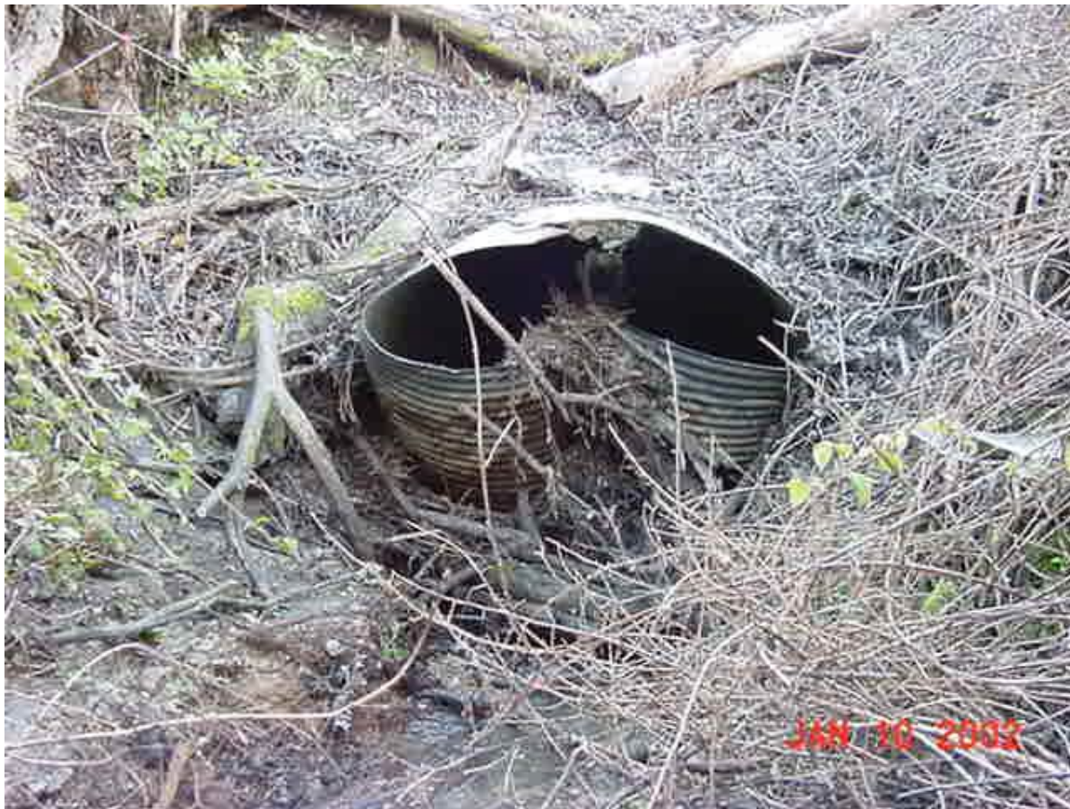
Photo 15 – Photo of 60-inch CMP culvert inlet at the Bear Gulch Road project site. Storm events in 1998 along with natural wearing resulted in a partially crushed inlet and damages throughout the pipe. Picture was taken in January 10, 2002. Clear Creek stream flows have navigated around the inlet and flooring and have gradually dissolved the road fill material. Natural woody debris and substrate movement within the stream is greatly hindered by the condition of the existing culvert. Note the woody debris accumulation on and around the culvert.
