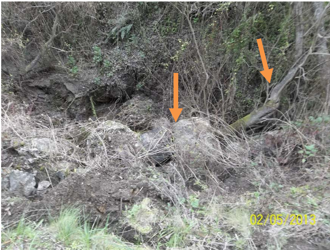
Photo 14 – Photo of slipped materials in the unnamed tributary channel. Arrows indicate location of slipped boulders and the undermined willow. The boulder and tree were removed from the entrenched channel to prevent flooding from upcoming rain events. The stream’s confluence with San Gregorio Creek is approximately 100 feet downstream of the slip-out #2 and 50 feet downstream of slip-out #1.
