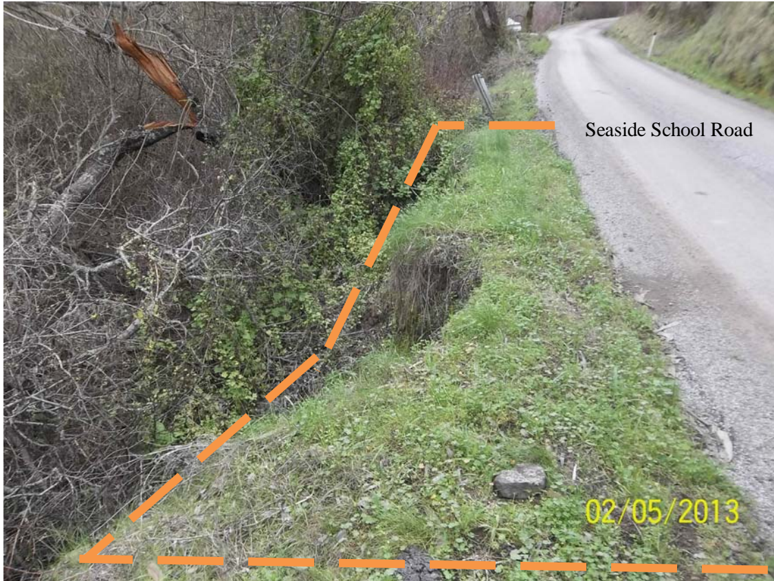
Photo 13 – Photo of slip-out location in relation to Seaside School Road. In the past, emergency repairs were completed to repair a slip-out at the same location. Recently an undermined willow tree fell from the road shoulder and caused another slip-out. Dashed lines indicate expected area of disturbance and previous extent of shoulder.
