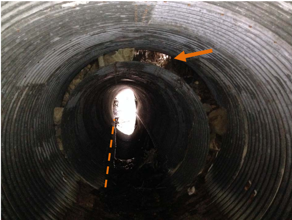
Photo 17 – Photo of culvert inlet showing disconnection of a 20-foot section of culvert inlet from the remaining pipe. Total loss of culvert flooring within this 20-foot section has caused the pipe to fully disconnect from the remaining pipe, reducing the volume carrying capacity of the pipe and causing the fill around the pipe to sink. Dashed line indicates location of the 20-foot section of pipe. Note the light entering the culvert from the earth fill as indicated by the arrow. The sinkhole is situated on top of the fill around the disconnected section of pipe.
