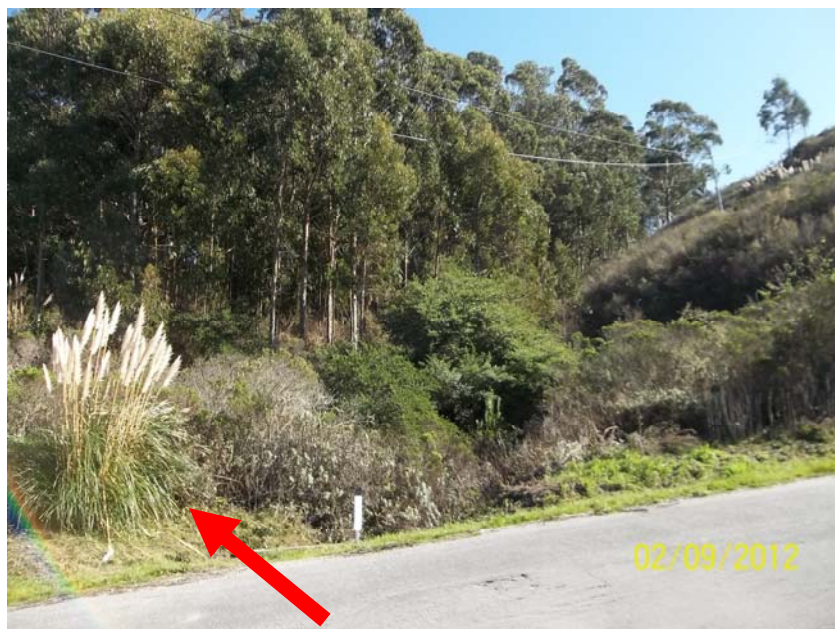
Photo 28 – Photo of drainage and eucalyptus grove on culvert inlet. Pampas grass individual to the left of the white culvert marker will be removed.
