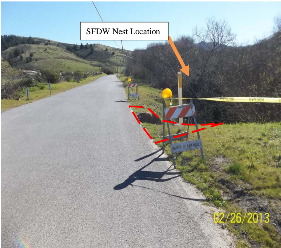
Photo 3 - Photo of slip-out looking east on Higgins Canyon Road. Dashed lines indicate immediate construction area. Slip-out deteriorated from the edge of pavement and eroded into the channel. Location of San Francisco dusky-footed woodrat nest location indicated by arrow.
