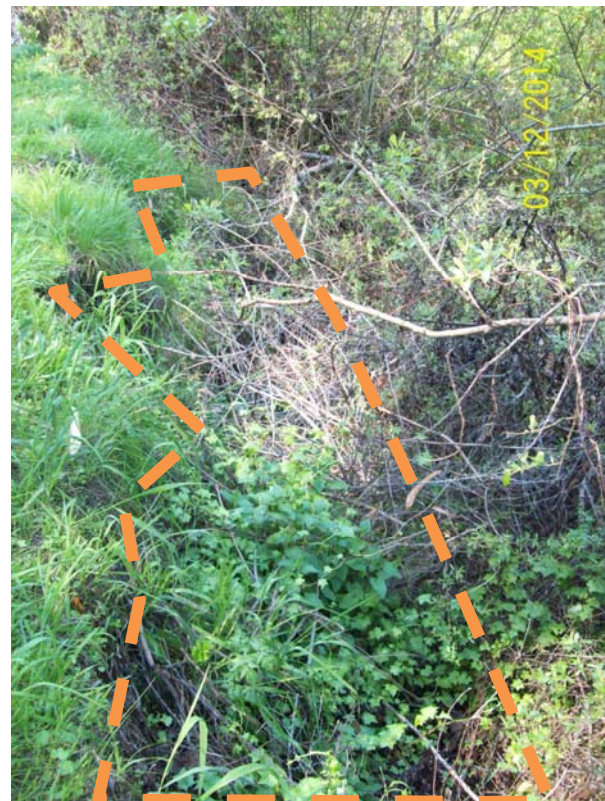
Photo 11 – Photo of slip-out looking west from Seaside School Road. Only herbaceous vegetation (cape ivy, miner's lettuce, milk thistle, bed straw) exists in the slipped material. The overhanging vegetation will need to be thinned to provide construction access and visibility of the slipped area. Dashed lines indicate slip-out location and previous extent of
