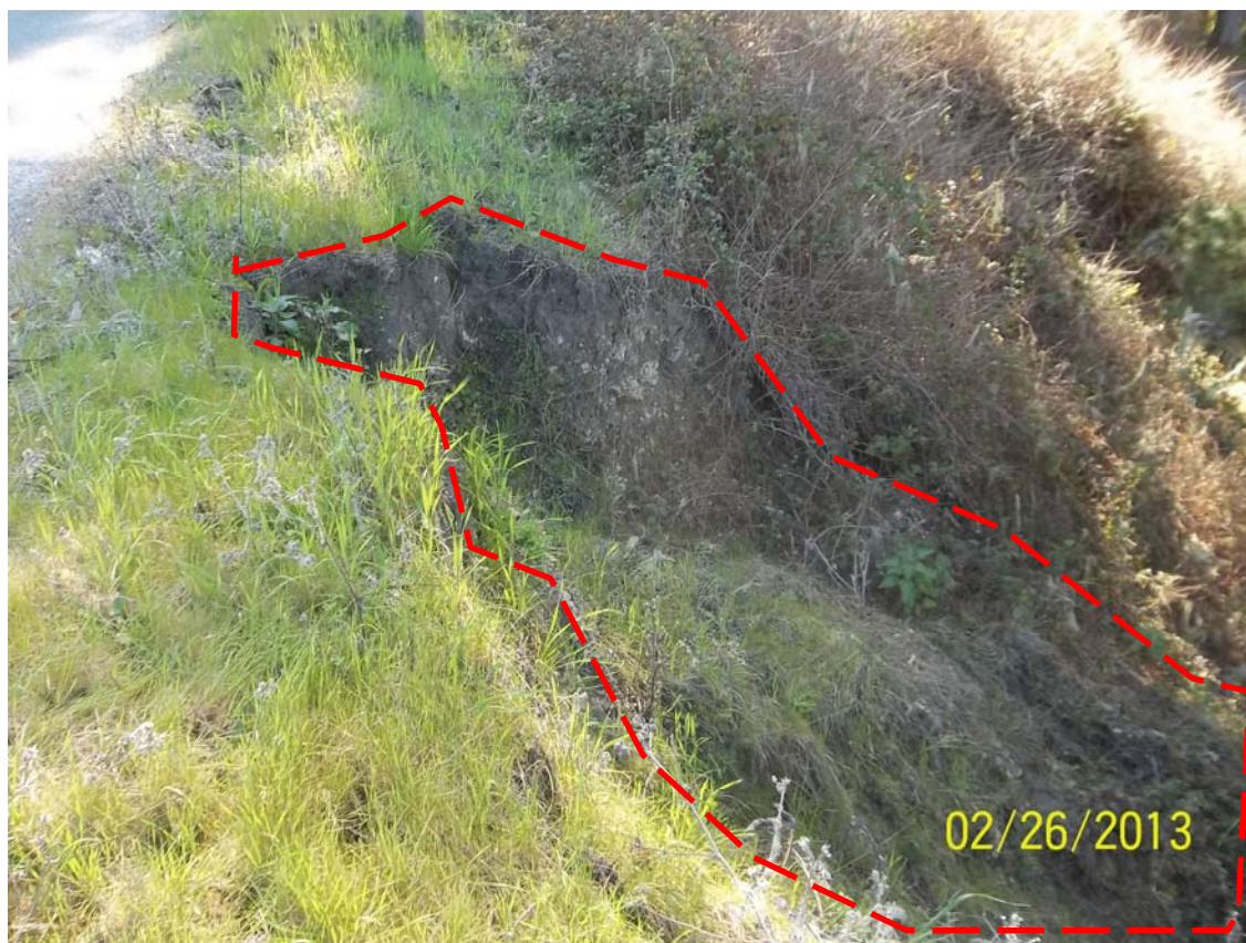
Photo 6 – Photo showing the extent of the slip-out indicated by the dashed lines. Damage caused by voles is prevalent throughout the shoulder. Cause of slippage might be due to a combination of factors including but not limited to vole burrows, unnatural consolidation of water run-off, and roadside vegetation management.
