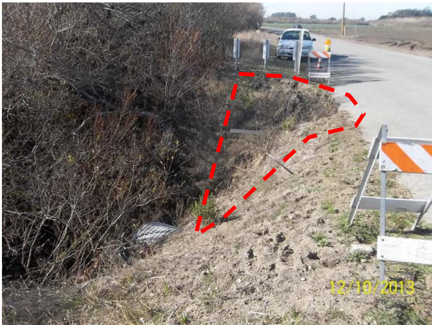
Photo 2 - Photo of slip-out dated December 10, 2013. Most of the annual grasses have died or eroded into the drainage revealing more of the damaged shoulder. Three reflector posts have been installed to reduce the possibility of motorists inadvertently driving into drainage. Dashed lines indicate the location of the slip-out. Note the erosion has reached the edge of pavement; whereas the edge of pavement in Photo 1 is still protected by a sliver of dirt.
