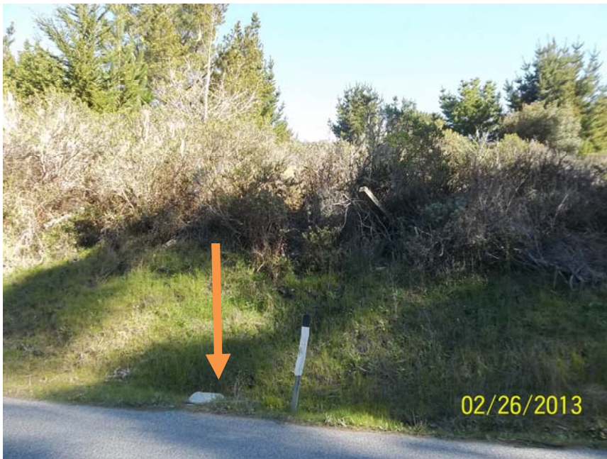
Photo 8 – Photo of 15-inch CMP culvert inlet along Higgins Canyon Road. The inlet drains the surrounding hillside and an earthen ditch. Parcel on upslope side of the road is part of Burleigh Murray Ranch State Park.
