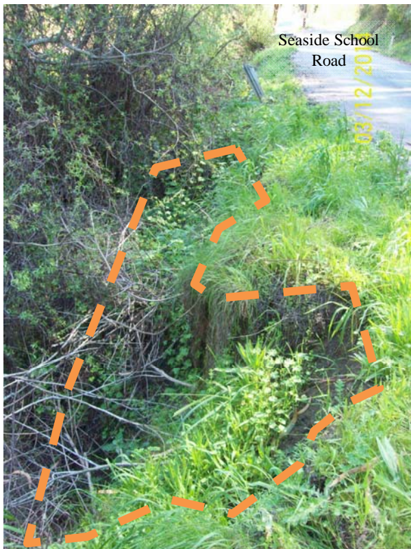
Photo 10 – Photo of slip-out looking east from Seaside School Road. Slipped soils were not observed in the channel or in the slipped area, indicating that past streamflows have transported the material downstream. Dashed lines indicate slip-out location and previous extent of shoulder.
