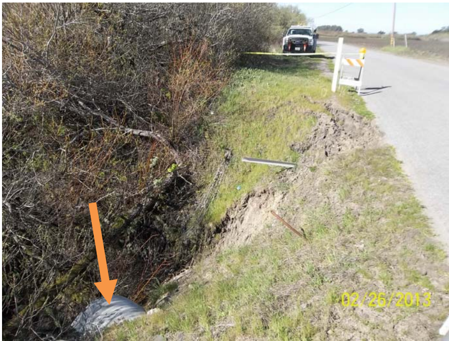
Photo 1 - Photo of slip-out dated February 26, 2013. Several shallow-rooted annual grasses visible on shoulder and in slipped area. The 36-inch culvert outlet is visible on bottom left corner of picture as indicated by the arrow.
