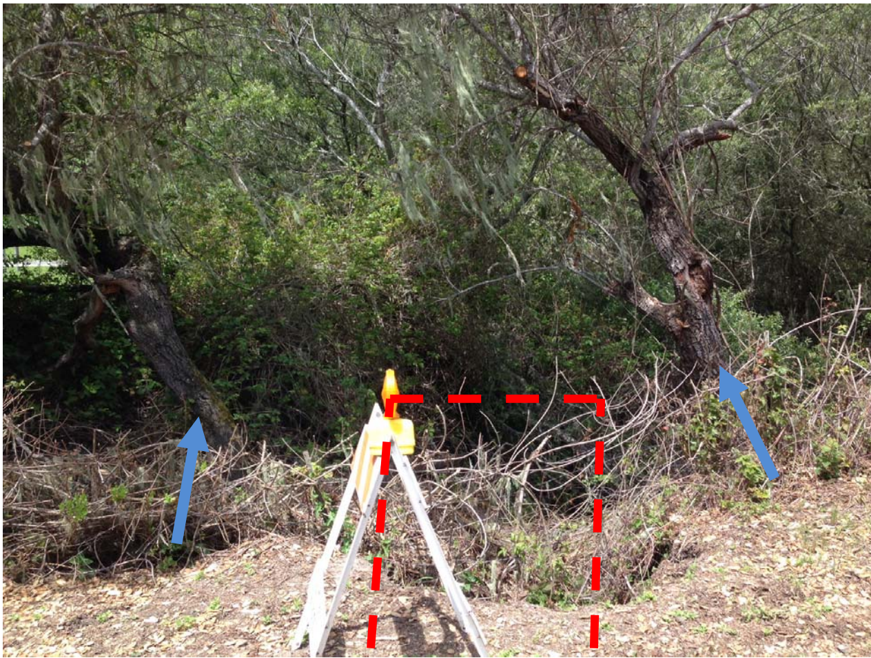
Photo 21 – Photo of culvert inlet with the two arroyo willow trees proposed for removal. Tree diameters are approximately 12- to 13-inch at breast height. Removal of the trees is necessary to extract the failing culvert as their trunks and roots exist within directly over and adjacent to the culvert. Trees will not be removed if determined unnecessary during the construction process. Dashed lines indicate approximate location of culvert in relation to the arroyo willow trees.
