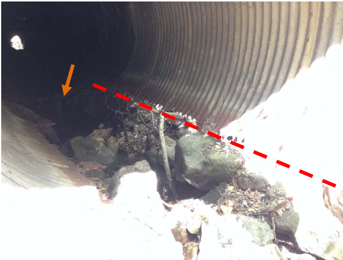
Photo 16 – Photo of 60-inch CMP culvert outlet showing fully deteriorated culvert flooring. Dashed line indicates downstream extent of culvert flooring loss. Arrow indicates downstream extent of remaining but deteriorated culvert flooring. Culvert outlet is perched at least 3 feet from the streambed. Moreover, the deteriorated flooring and stream flow around the pipe has resulted in loss of road fill at the outlet and inlet. Surface flow was absent during the December 2013 and February 2014 visits but minor surface flow was present during the March 2014 visit. Construction will take place when surface flow is absent and the appropriate permits have been obtained.
