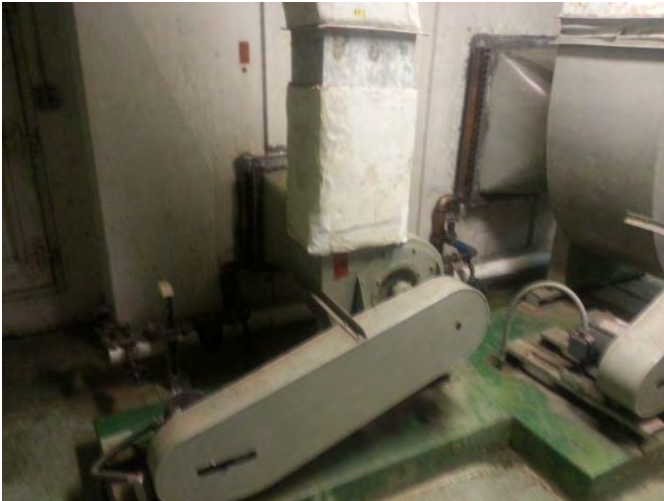
Photo M-5 – Supply Fans
