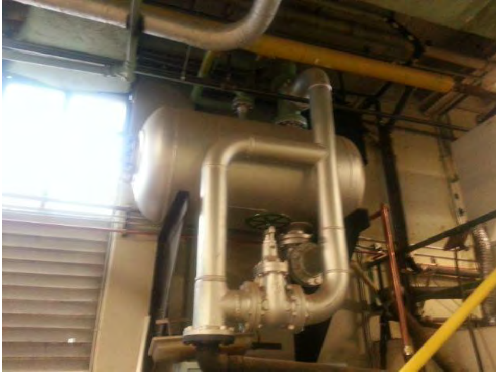
Photo M-4 – Flash Tanks
