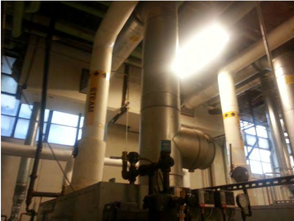
Photo M-2 – Boiler Flue
