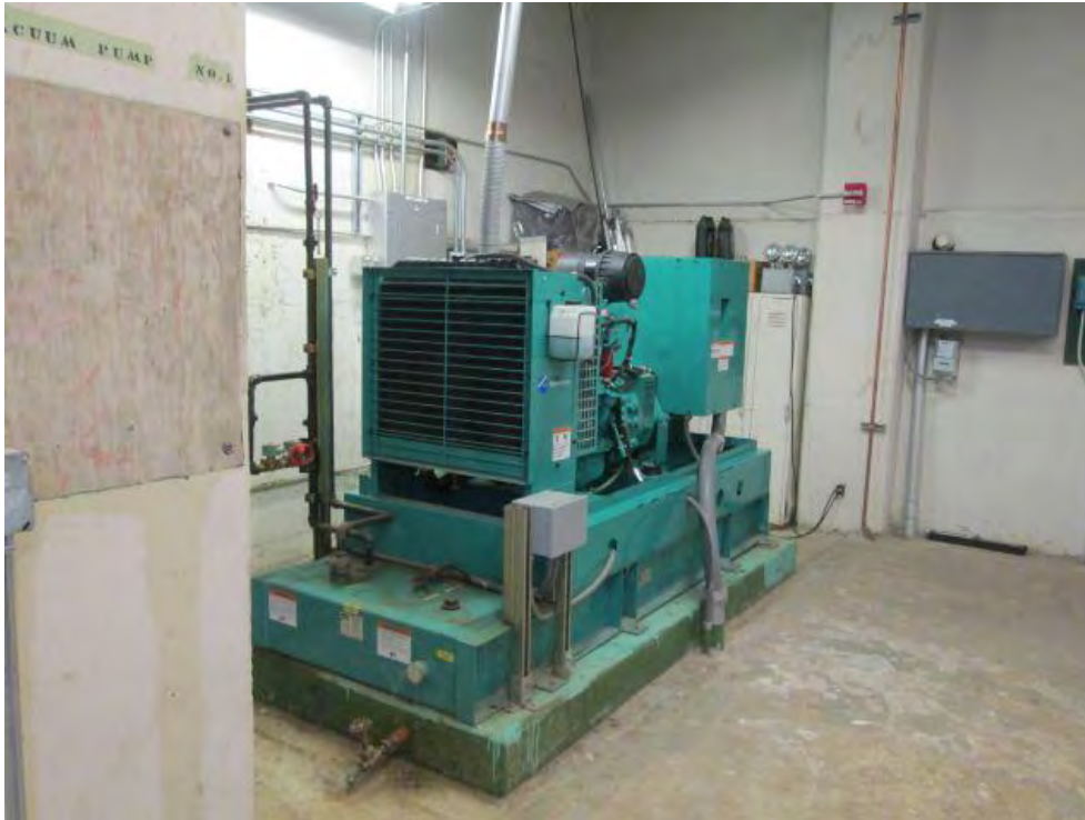
Photo E-1 - Genset
