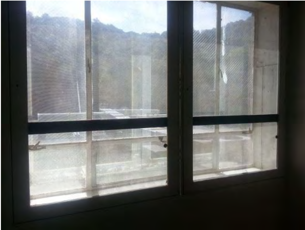
Photo M-6 – Operable Windows have been screened off due to security reasons.
