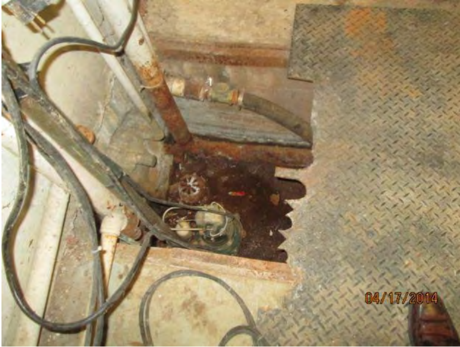
Photo P-5 - Sump Pumps in Trench
