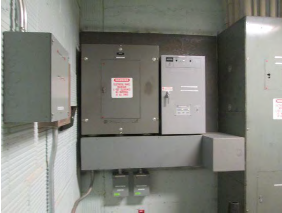
Photo E-7 - Electrical Panel
