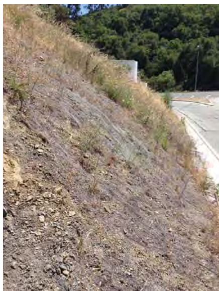
Photo 11: Cut slope at the junction of Edmonds Road and Edgewood Road composed of disintegrated sandstone and shale
