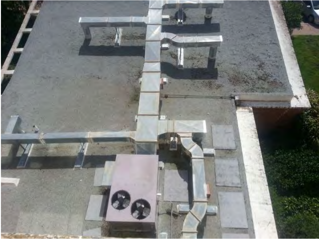
Photo M-10 – Roof Packaged Heat Pumps
