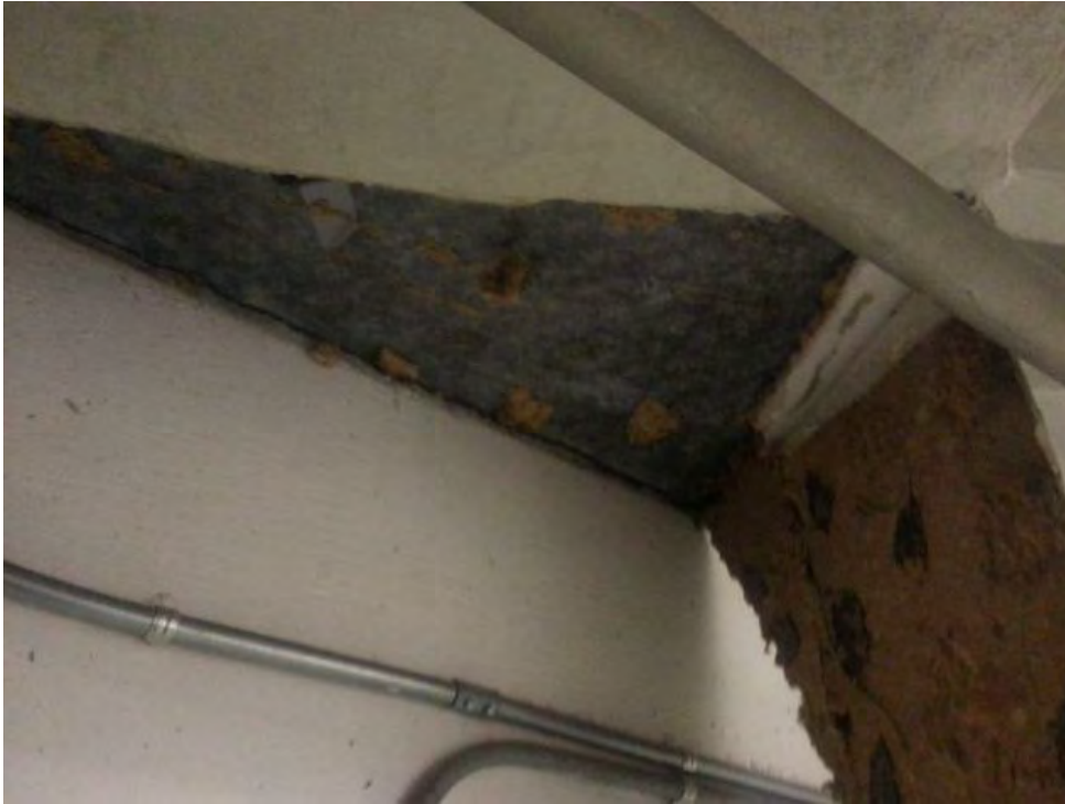
Photo M-8 – Duct Insulation
