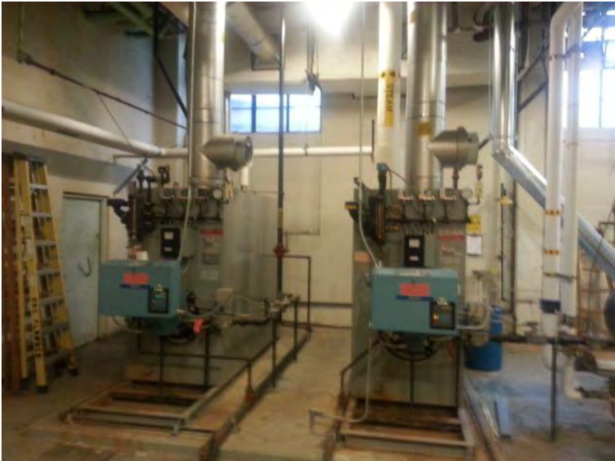
Photo M-1 - Boiler
