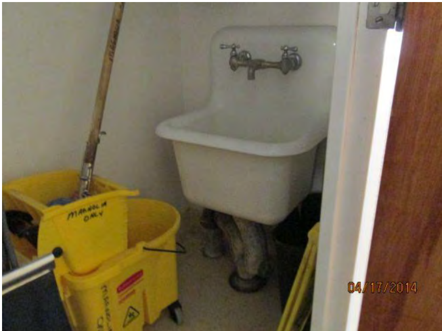
Photo P-3 - Outdated Type of Janitor Sink
