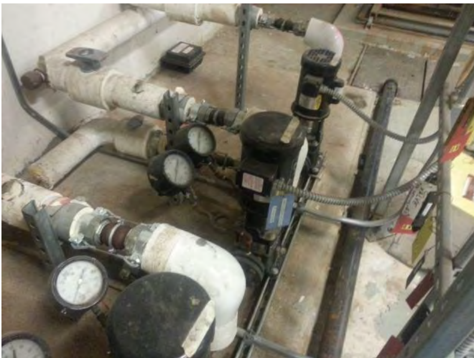
Photo M-3 - Pumps
