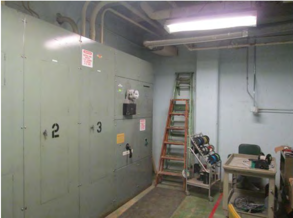
Photo E-5 -Main Switchboard
