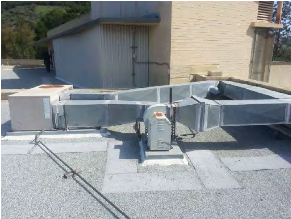
Photo M-9 – Roof Packaged Heat Pumps
