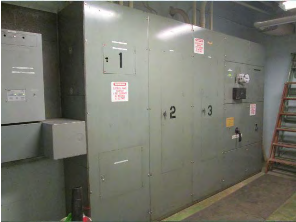
Photo E-6 - Switchboard
