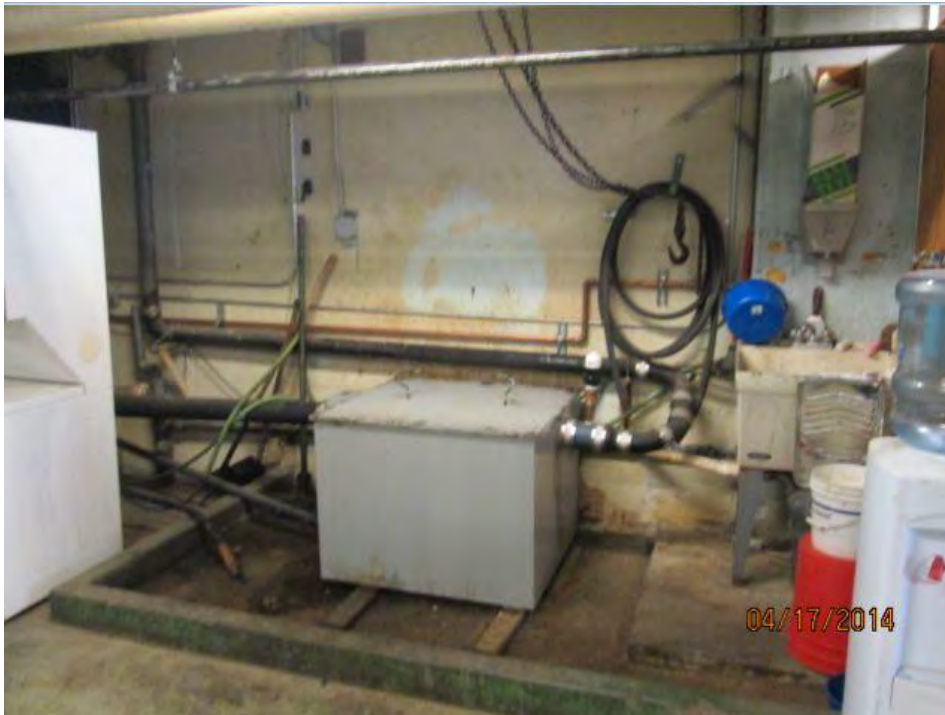
Photo P-1 - Grease Interceptor
