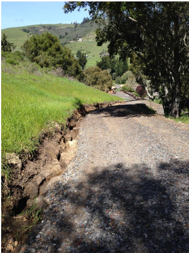
Erosion to be addressed in management plan
