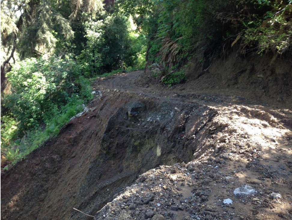
Slope instability to be addressed in management plan
