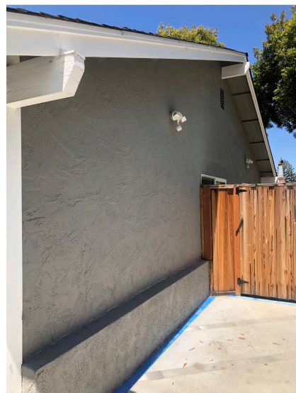
South side of the structure. (parking space on Alameda de las Pulgas)
